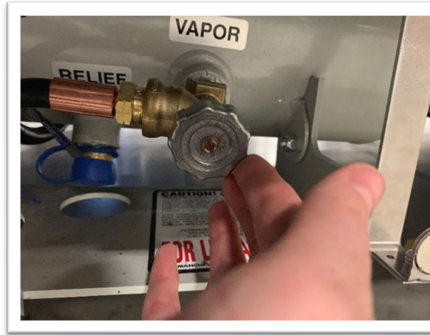
Propane tank main shutoff valve
