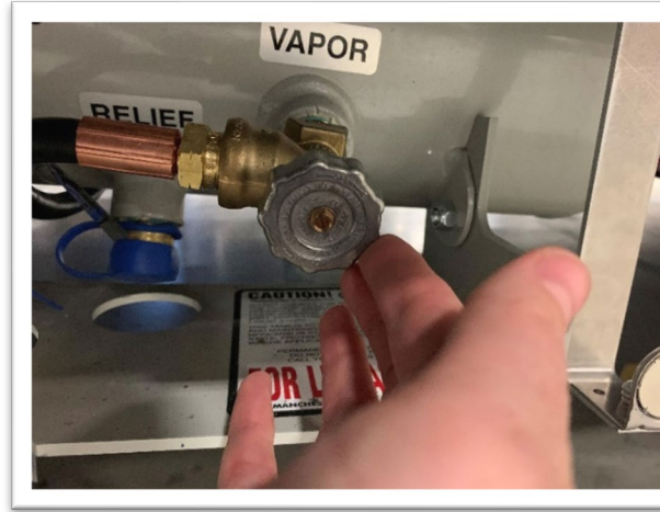
Propane tank main shutoff valve
