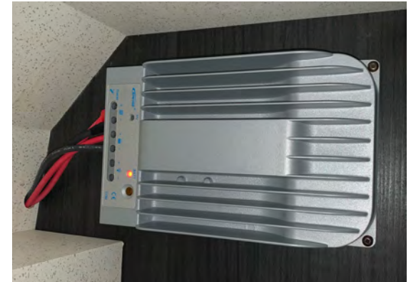
Picture 38.1 Solar charge controller
