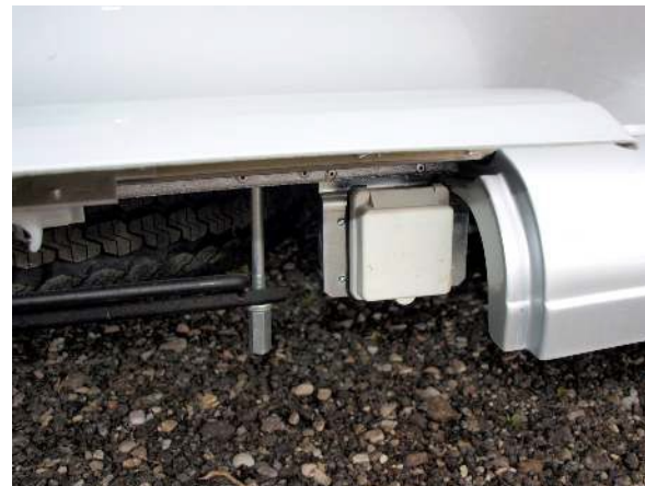
Shore Power connection point
