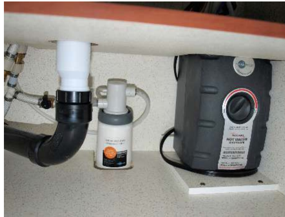
On demand hot water system filter
