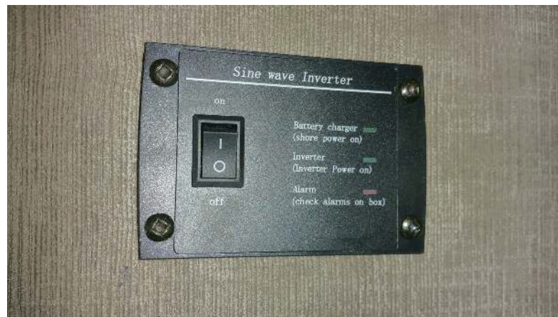
Inverter Control Panel
