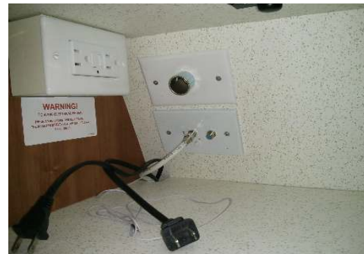
TV antenna and cable connections
