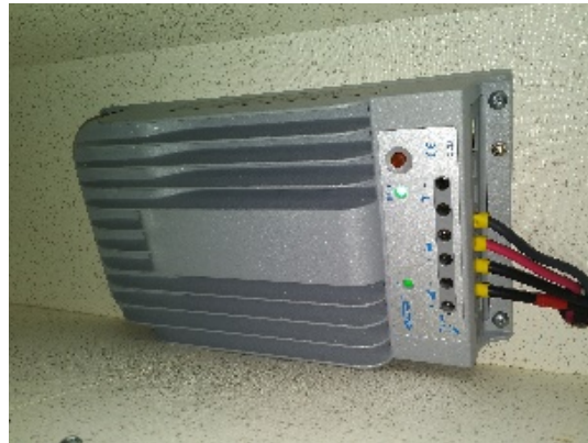
Solar controller in cabinet above galley
