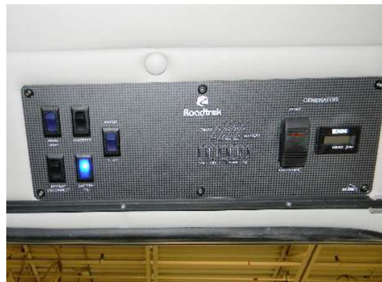
Monitor panel for units propane generator
