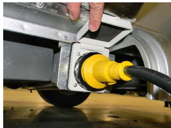
Attached shore power cord
