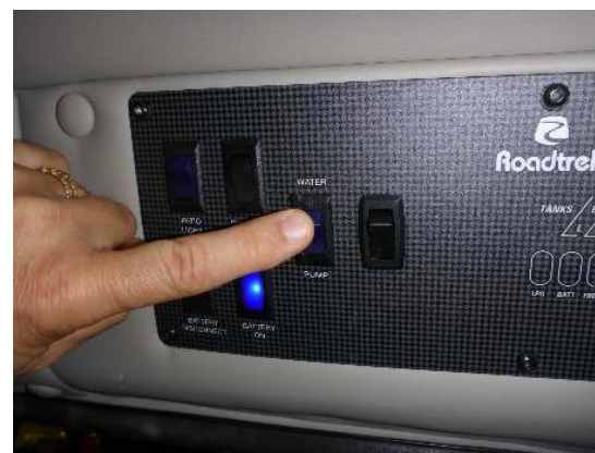
Picture 42.2 Water pump switch
