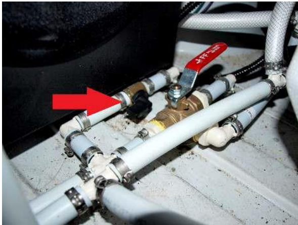
Tank isolator valve shown in open position (black plastic handle horizontal pointed along the water line)
