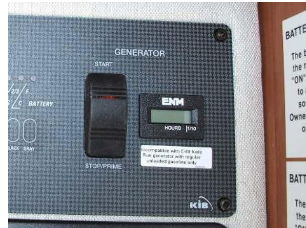
Generator switch and hour meter
