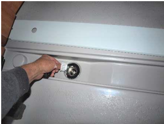
Aisle shower drain
