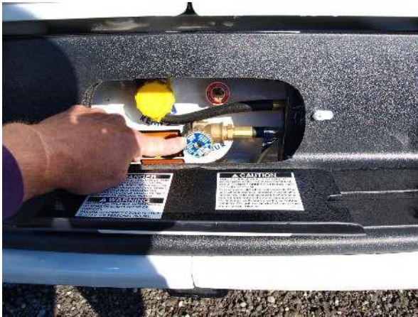
Propane tank main shutoff
