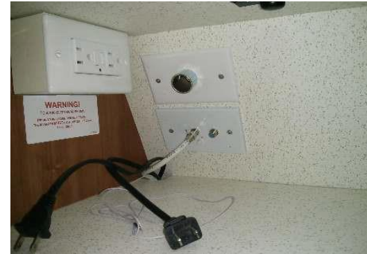
TV antenna and cable connections
