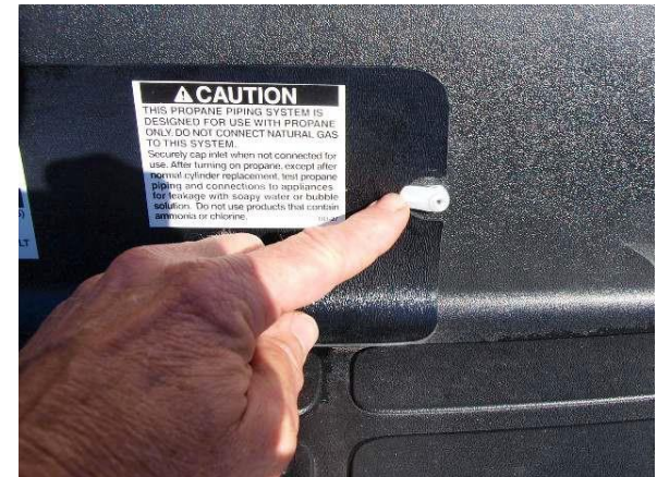
Propane access cover
