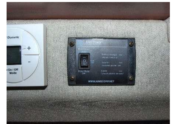
Inverter switch for optional 2500 watt inverter
