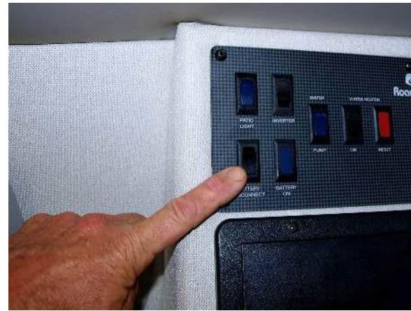
Battery disconnect switch
