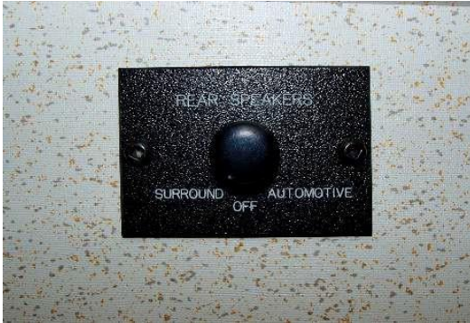
Rear speaker control switch
