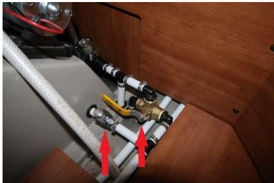
Tank selector valve in exterior tank position
