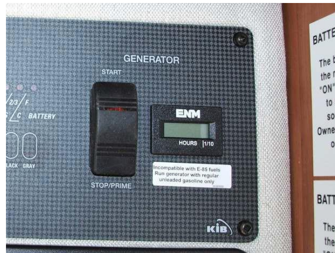
Generator switch and hour meter
