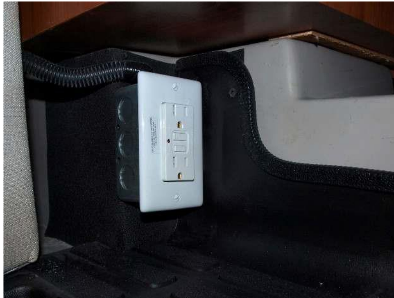
GFCI outlet under rear passenger side seat
