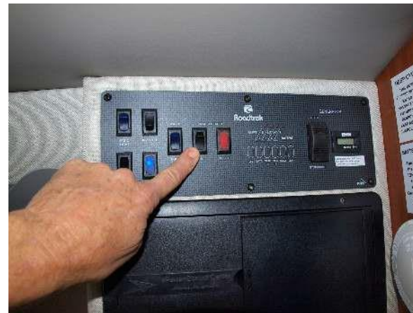
Water heater switch
