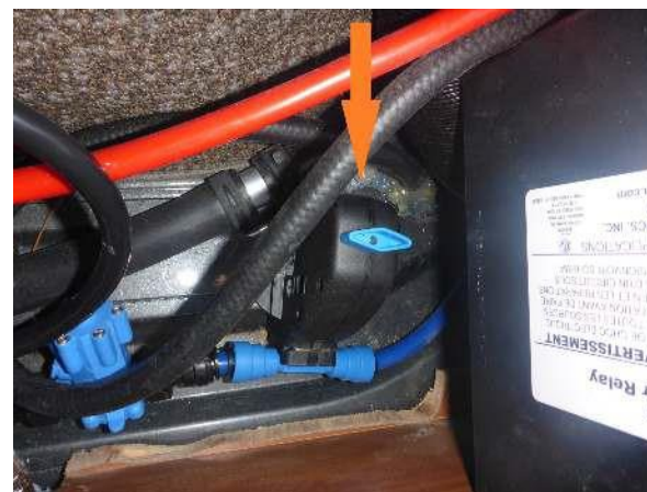
Resetting the tripped valve
