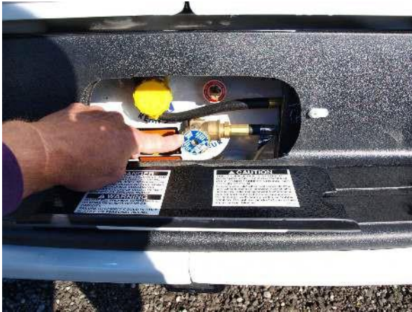
Propane tank main shutoff
