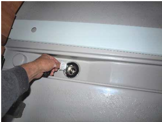
Aisle shower drain
