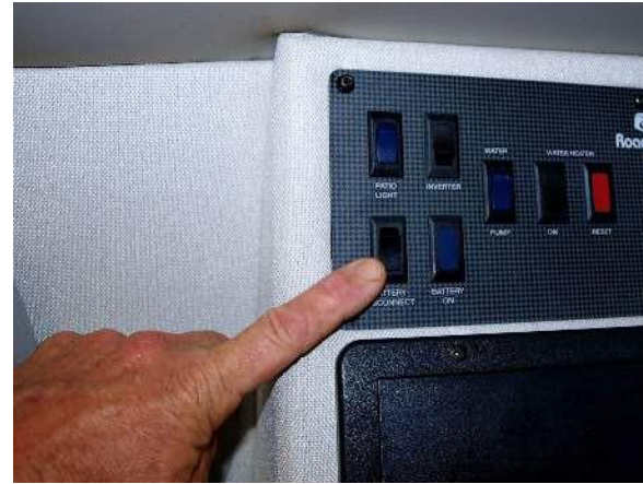
Battery disconnect switch
