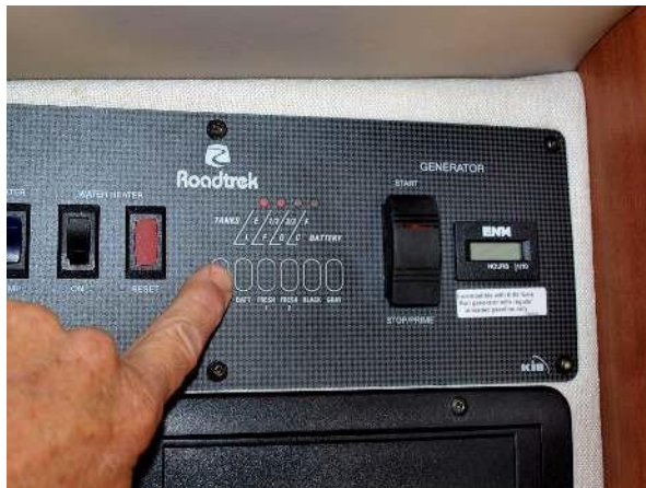
Tank status lights
