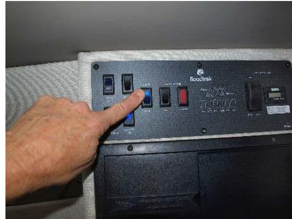
Water pump switch
