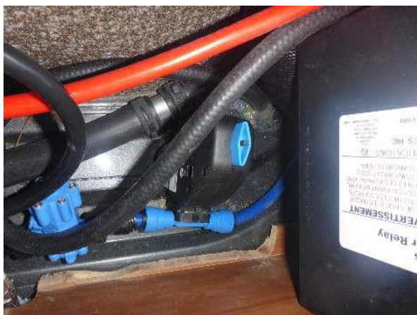
Alde frost control valve in operating position
