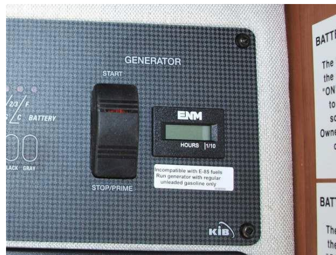
Generator switch and hour meter
