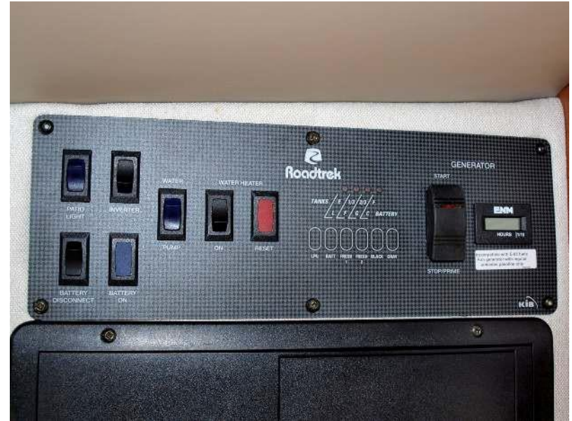
Monitor panel with standard 750 watt inverter and optional gasoline generator
