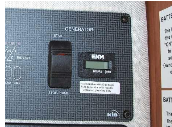
Generator switch and hour meter
