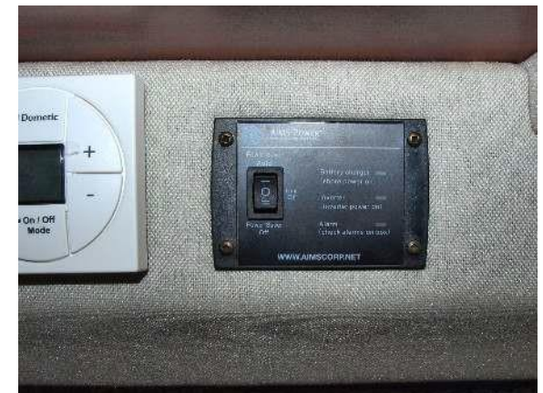
Inverter switch for optional 2500 watt inverter
