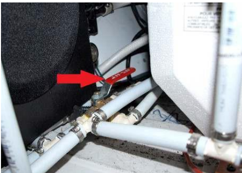
Tank selector valve in exterior tank position
