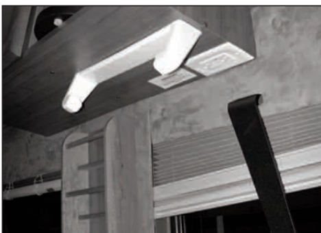
Picture E-P0A: 110V GFCI receptacle, (Galley location).
