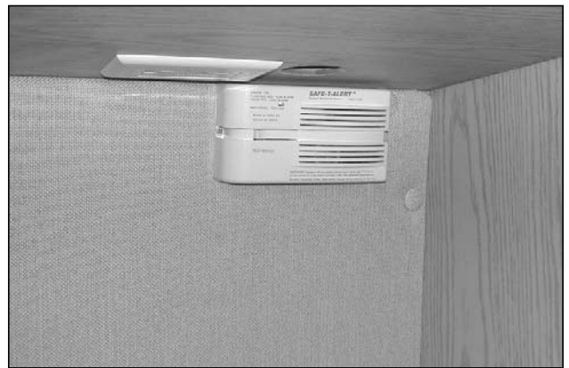
Picture F-P2: Carbon monoxide leak detector.
