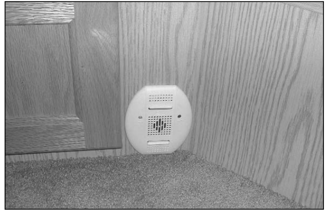
Picture F-P1: L.P.G. leak detector.
