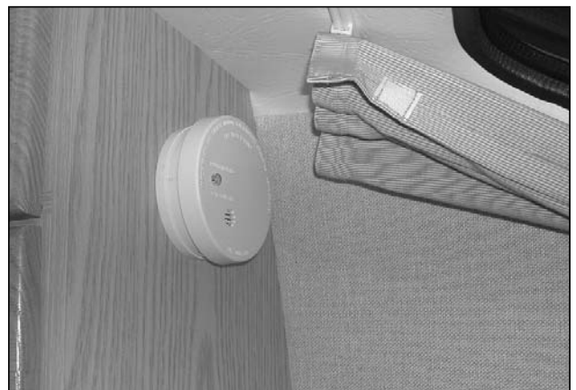
Picture F-P3: Smoke detector.
