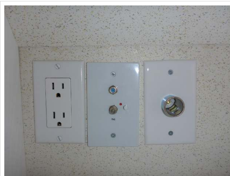
TV Antenna and Cable connections.
