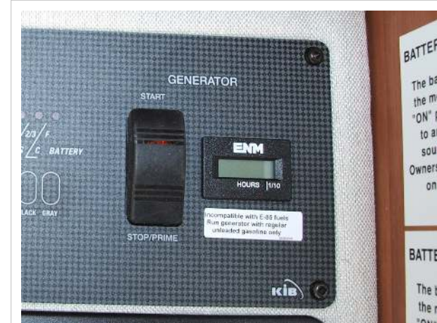
Generator switch and hour meter
