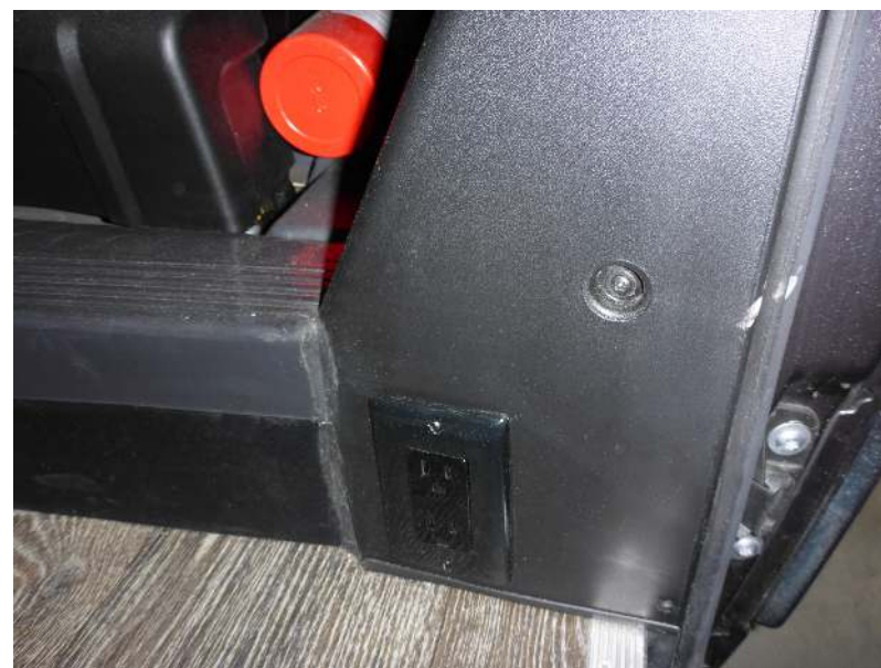
Outlet at side door
