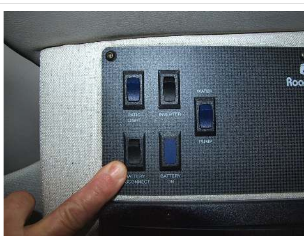
Battery disconnect switch
