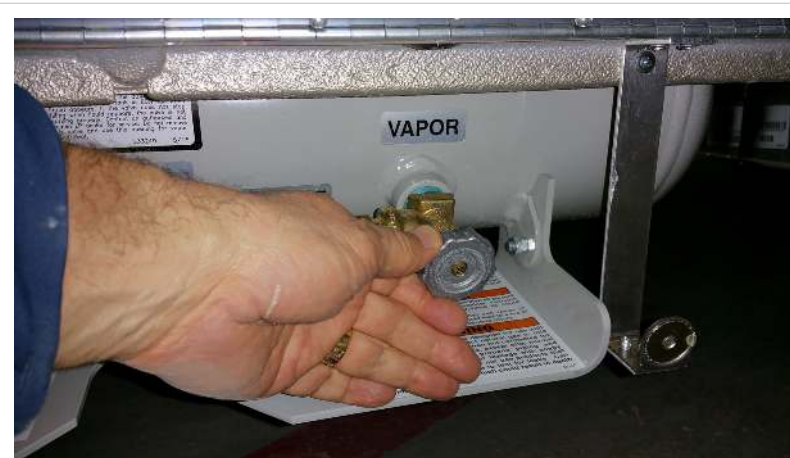
Propane tank main shutoff valve
