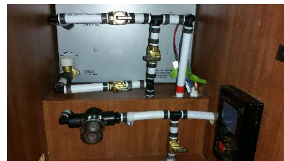
Tankless water heater drains
