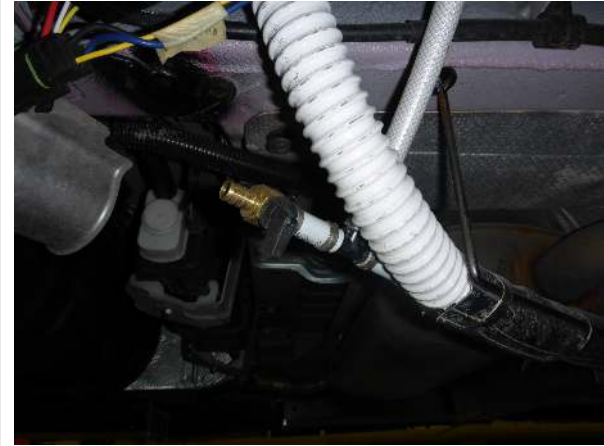
Tank drain, under driver's doorstep
