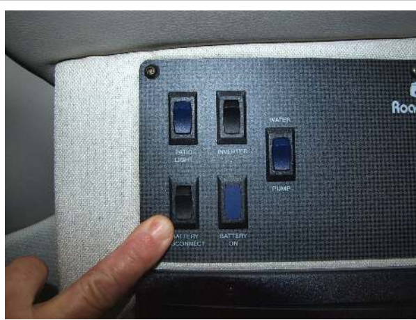
Battery disconnect switch
