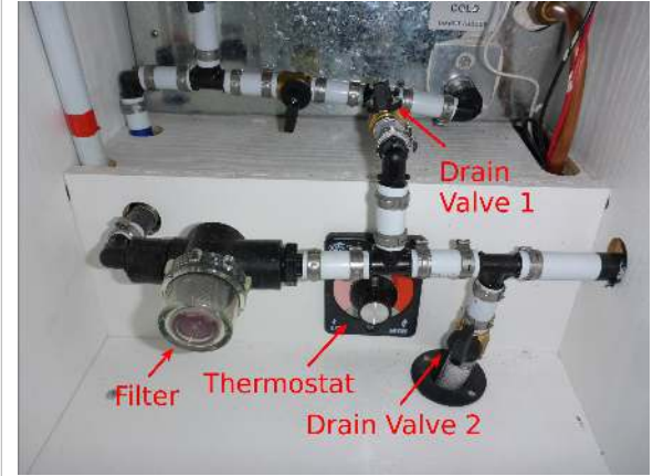
Tankless water heater drains
