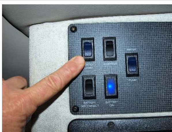
Patio light switch
