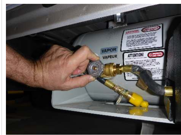
Propane tank main shutoff valve
