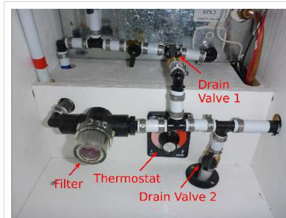
Water heater thermostat, filter and drain valves
