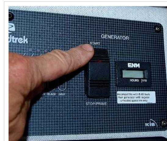
Starting the generator
