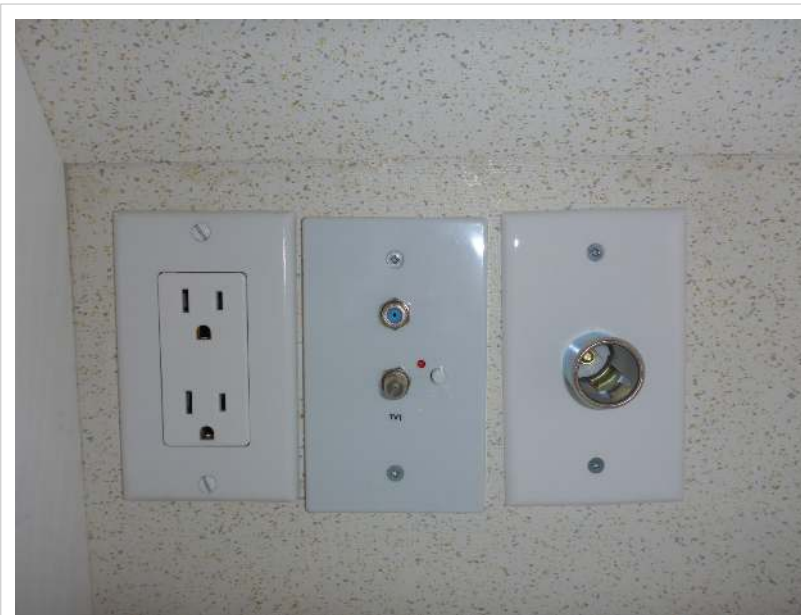
TV Antenna and Cable connections.
