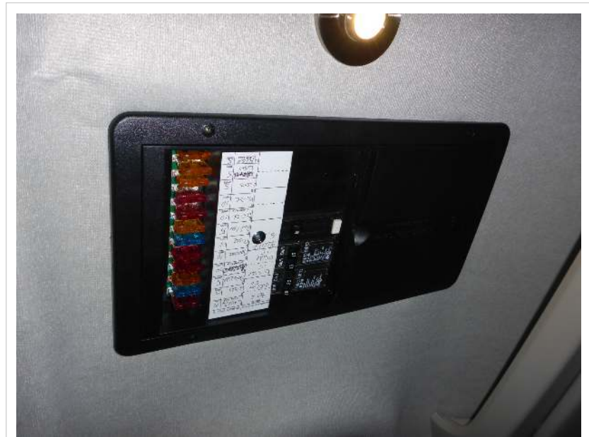
Breaker and fuse access
