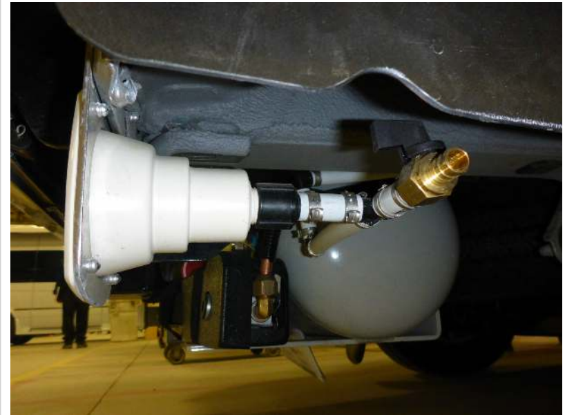
Rear drain behind the city water connection
