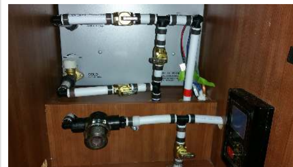
Tankless water heater drains
