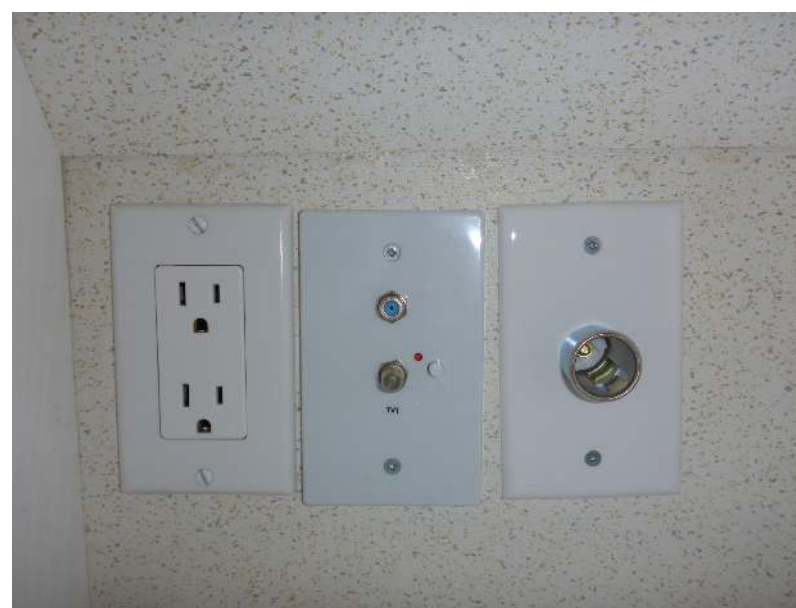
TV Antenna and Cable connections.
