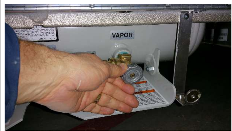
Propane tank main shutoff valve
