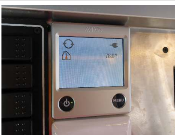
Alde control unit, in distribution panel
