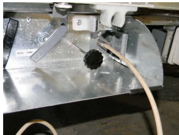
TV cable connected
