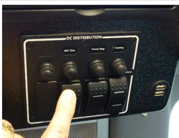
Battery disconnect switch
