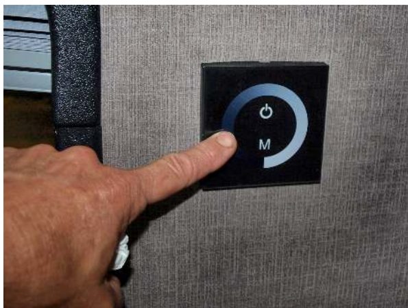
Strip light switch
