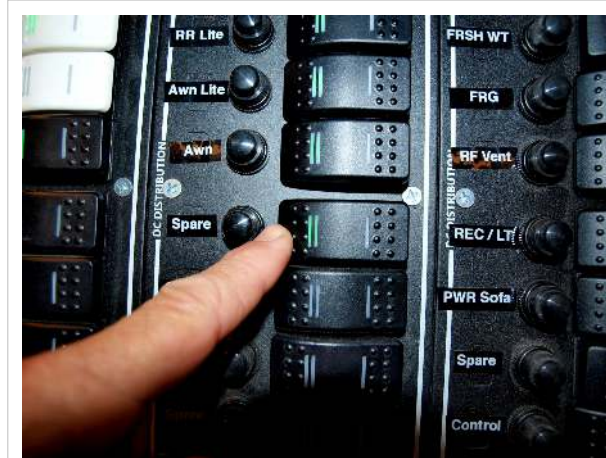
12 volt three-way switch in automatic position (two green lights illuminated)
