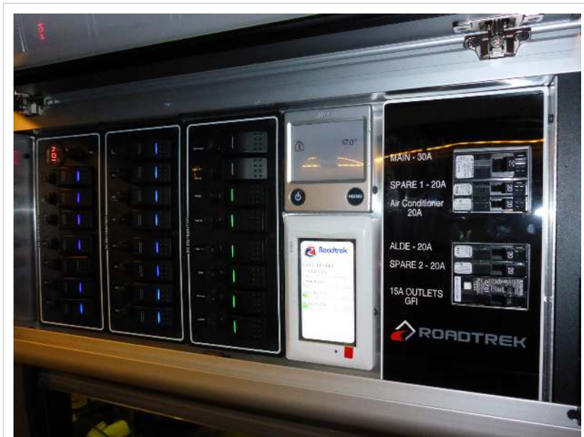
Distribution panel location, behind rearmost overhead cabinet door on drivers side; 120VAC breakers and labels on the right
