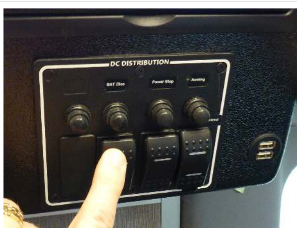
Battery disconnect switch
