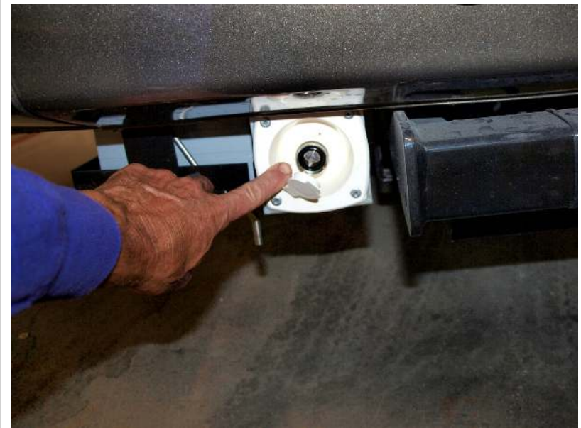
City water connection, on driver's side below rear bumper
