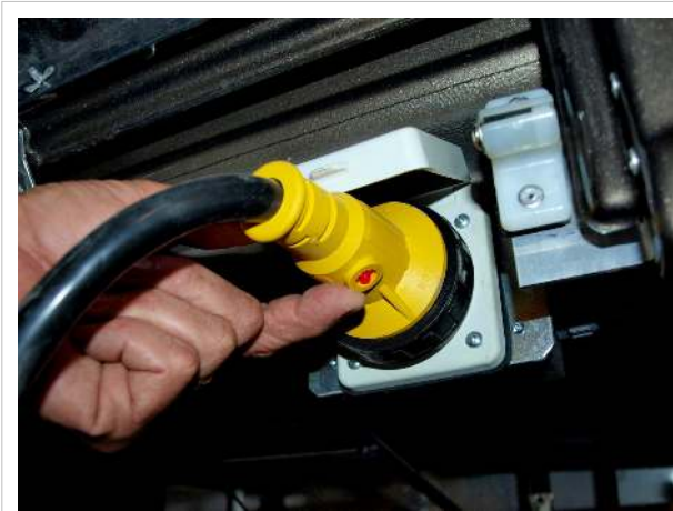
Some power cords have an LED on plug indicating shore power is being supplied
