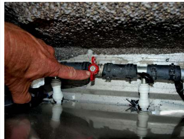
Valve to adjust floor heat, in full floor heat position
