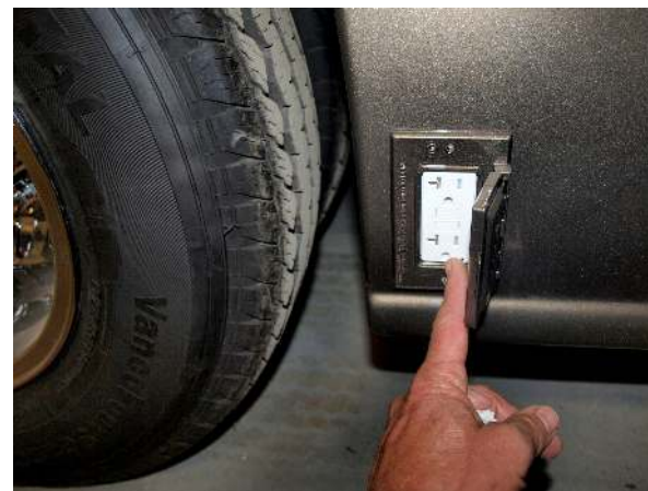
Outside electrical outlet
