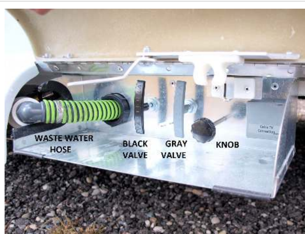
Waste water controls compartment_contents
