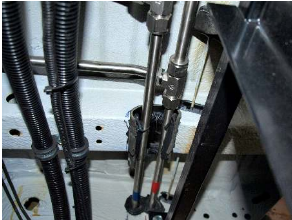
TS water lines underneath the floor
