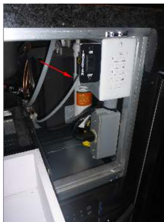
Unit and filter under counter
