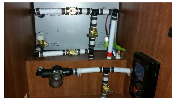
Tankless water heater drains
