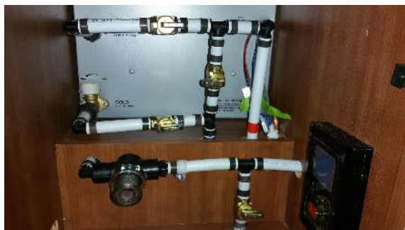
Water heater thermostat, filter and drain valves
