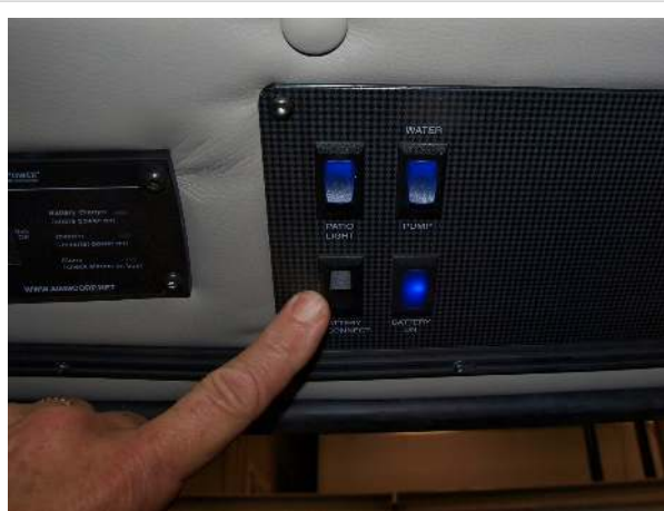
Battery disconnect switch
