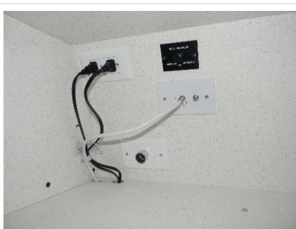
TV antenna switch and power injector
