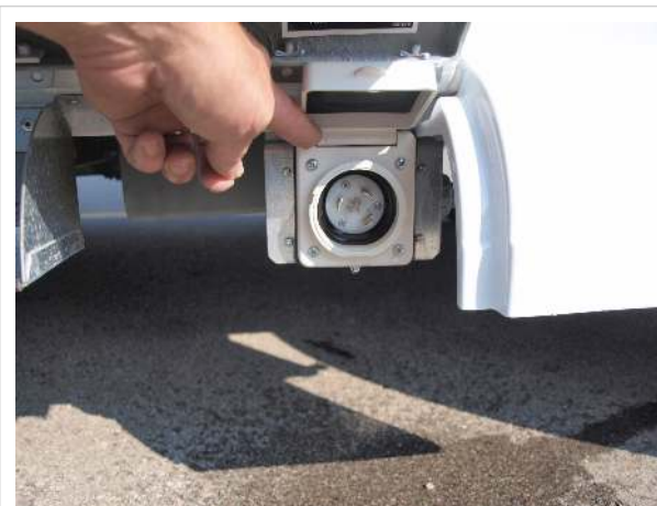
Shore power connection
