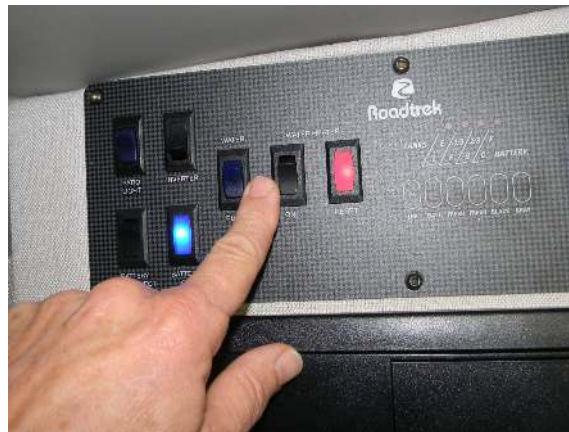
Water heater switch and red indicator light
