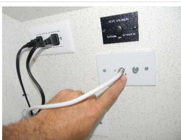
Antenna/cable AB switch
