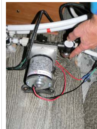
Water pump filter
