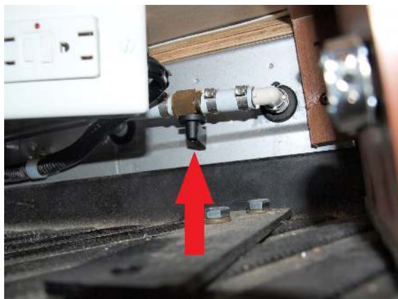
City water connection valve, shown closed
