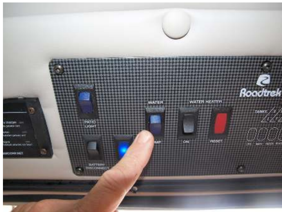
Water pump switch
