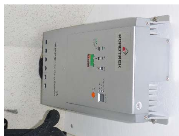
Solar controller in cabinet above galley
