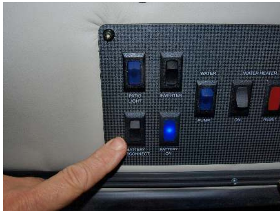
Battery disconnect switch
