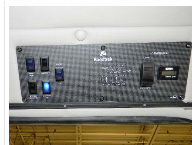
Monitor panel for units propane generator
