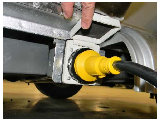
Attached shore power cord
