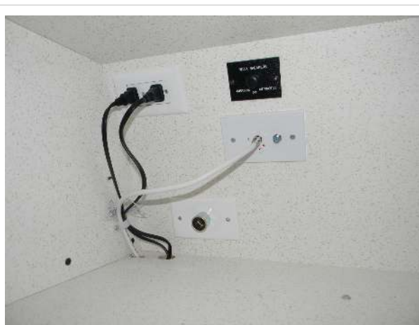
TV antenna and cable connections
