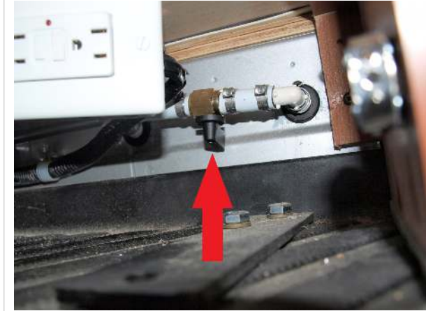
Closed city water valve (handle across line)
