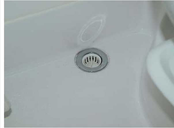
Shower floor drain plug
