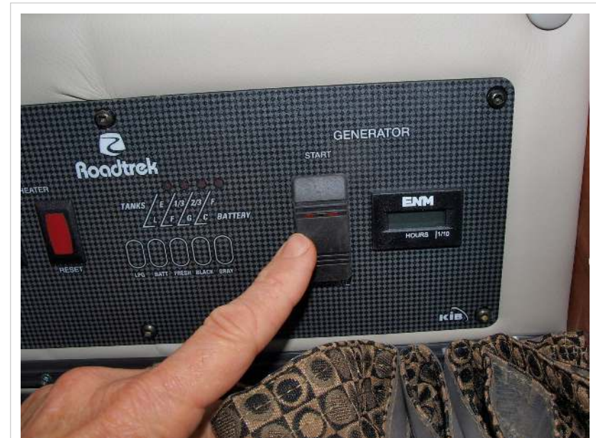
Generator switch and hour meter
