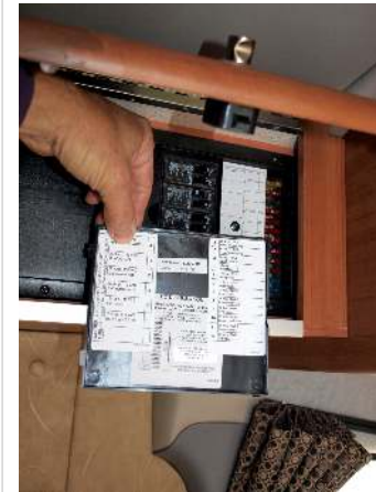
Agile AC breakers and 12 volt fuses
