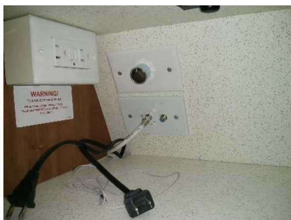
TV antenna and cable connections
