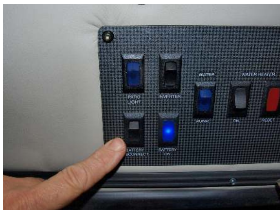
Battery disconnect switch
