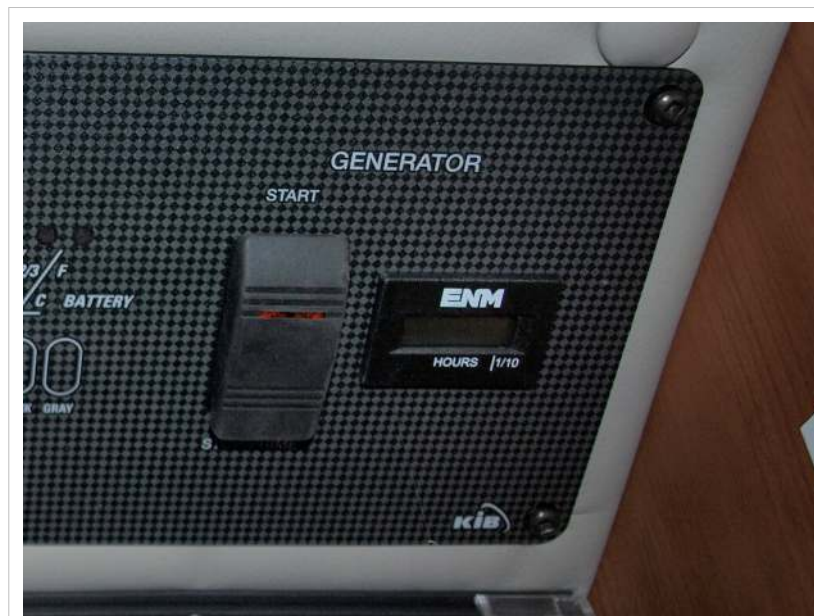
Generator switch and hour meter
