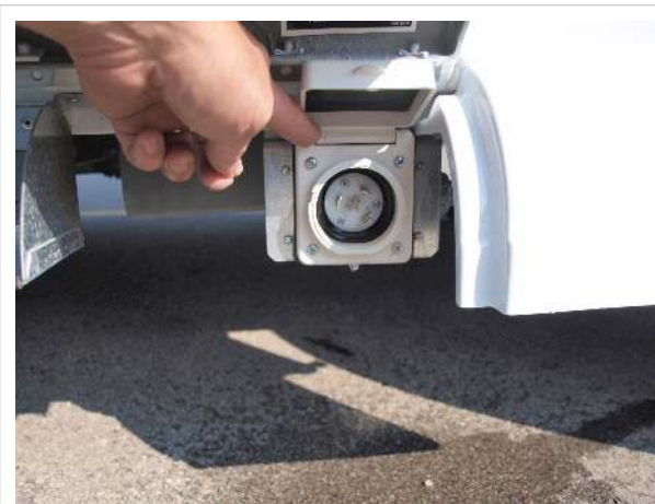
Shore power connection
