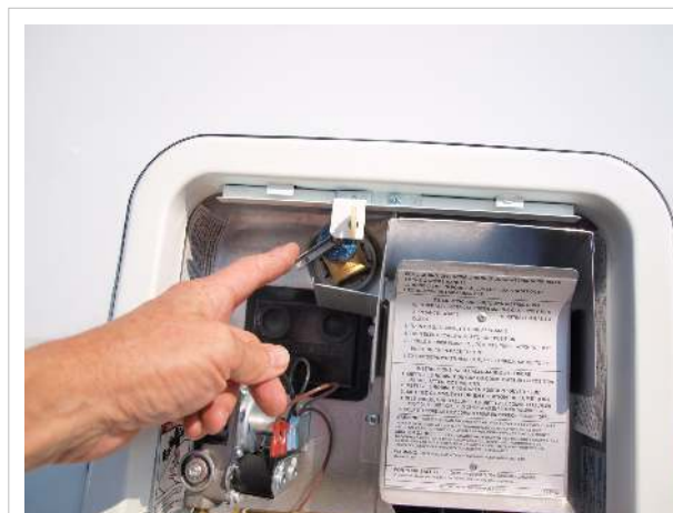
Water heater pressure relief valve
