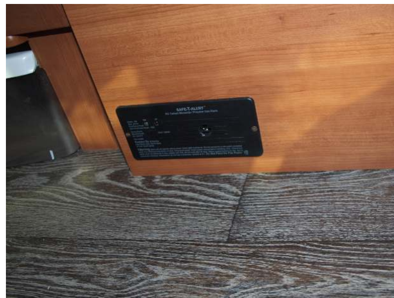
Propane and Carbon Monoxide alarm
