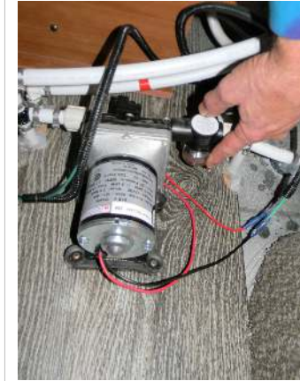
Water pump filter
