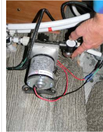
Water pump filter
