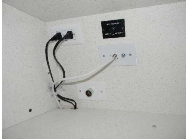
TV antenna switch and power injector
