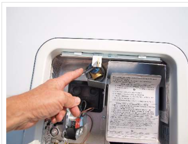
Water heater pressure relief valve
