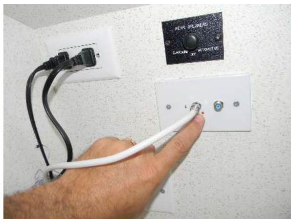
Antenna/cable AB switch
