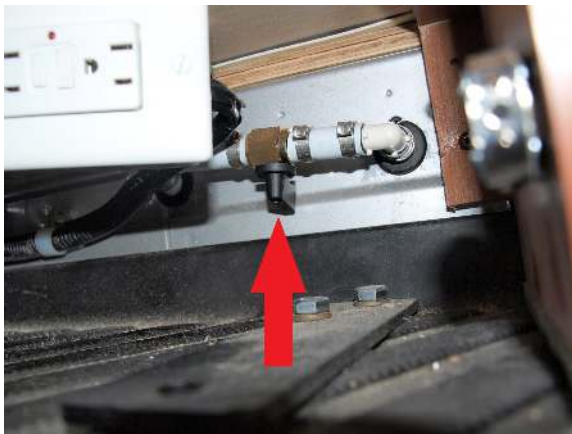
City water valve in closed (handle across the line) position
