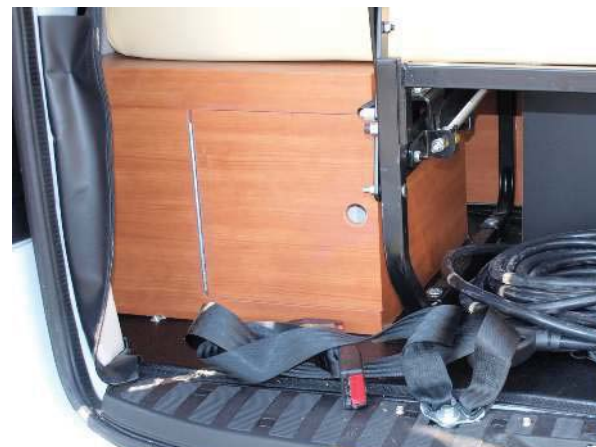
Water heater enclosure, under sofa and behind drivers side rear door
