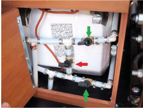
Water heater bypass valves in the normal position, all pointing to the left. Green means open, red closed.
