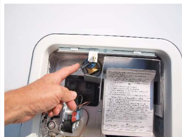
Water heater pressure relief valve
