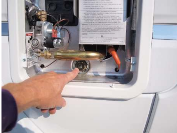
Water Heater Anode
