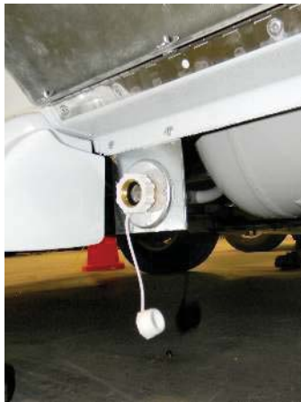
City water fill location
