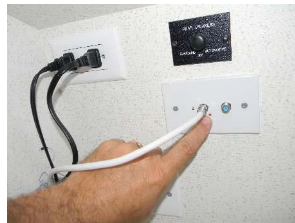
Antenna/cable AB switch
