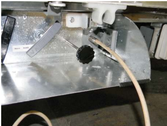
TV cable connected
