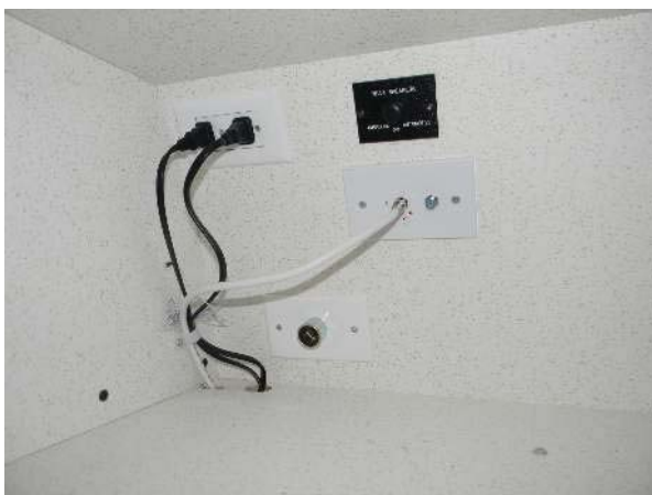
TV antenna switch and power injector
