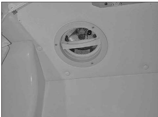
Picture B-P20: Bathroom exhaust vent.
