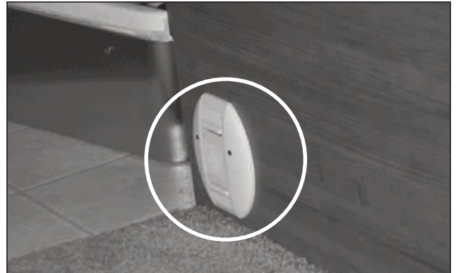
Picture F-P1: Propane leak detector.
