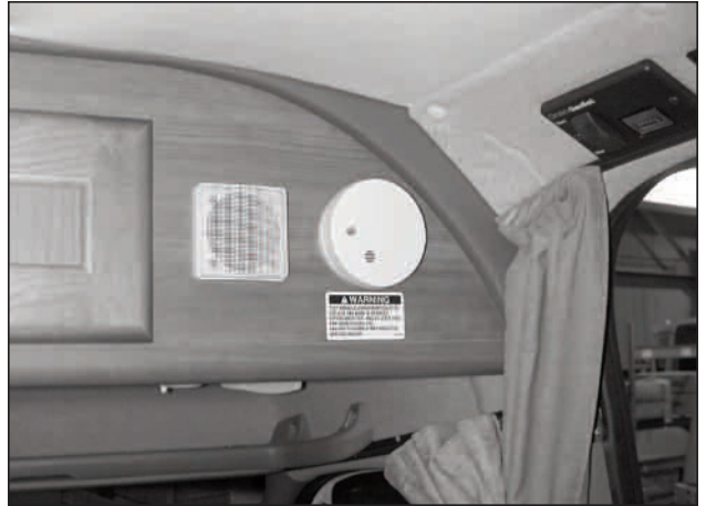
Picture F-P3: Smoke detector.
