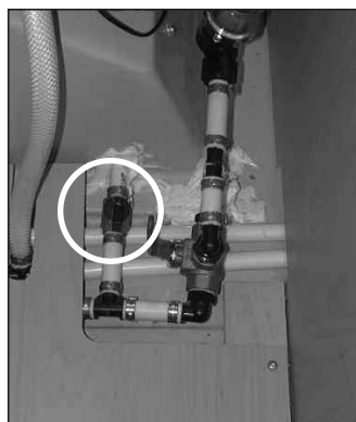
Picture G-P6a: Interior tank drain valve in open position.
