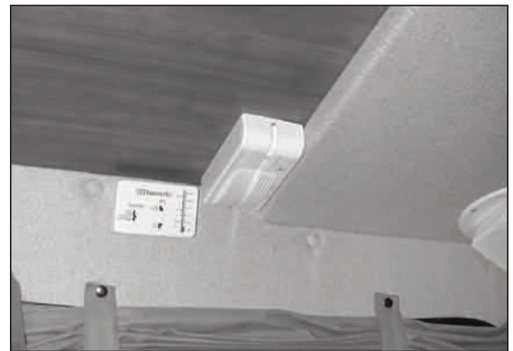
Picture F-P2: Carbon monoxide leak detector.
