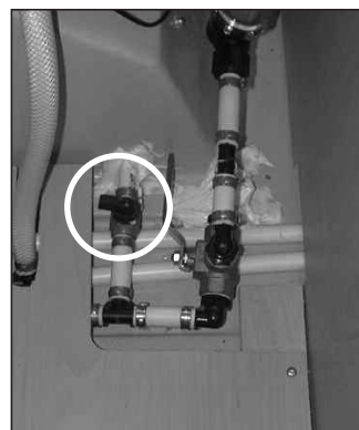
Picture G-P6b: Interior tank drain valve in closed position.
