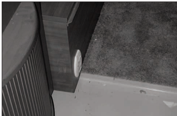
Picture F-P1: Propane leak detector.
