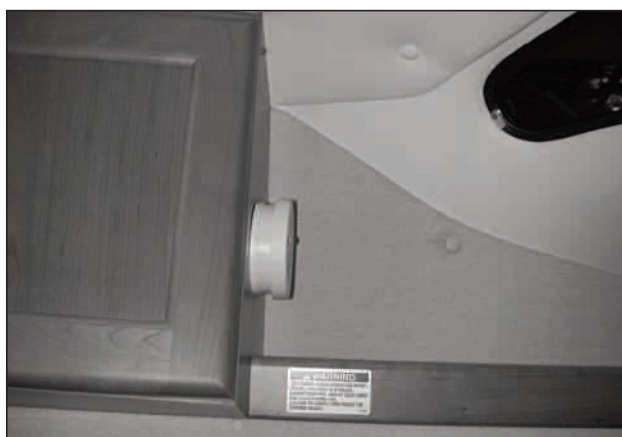
Picture F-P3: Smoke detector.
