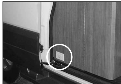
Picture E-P2: 110V GFCI receptacle, (side entry door location).
