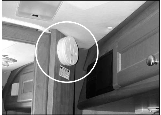
Picture F-P2: Smoke detector.
