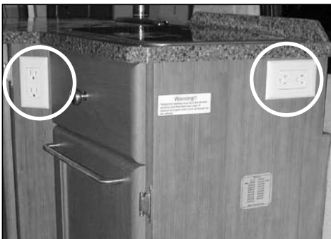
Picture E-P1: 110V GFCI protected receptacles, (Galley location).
