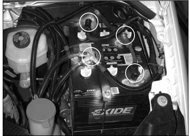
Picture B-P45: Auxiliary battery location showing cable connection hex nuts.
