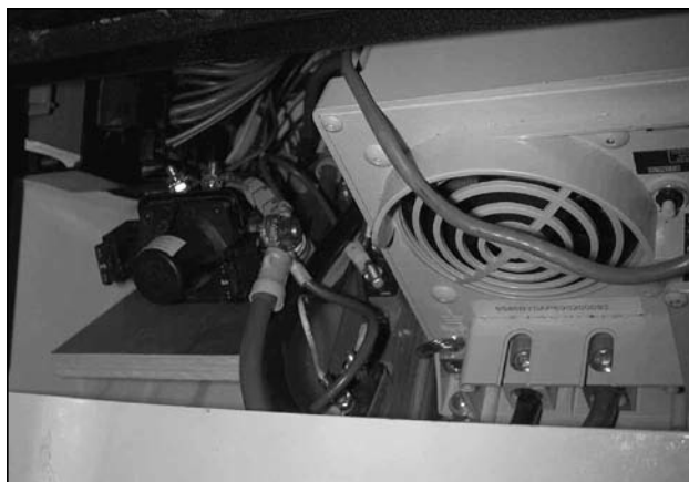
Picture I-P03: Location of 10 Amp slide out breaker.
