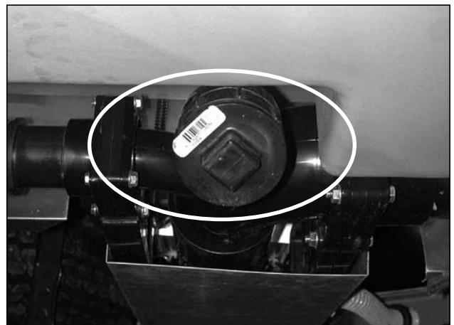
Picture G-P13: Sewage discharge manual cleanout.(As seen from below the vehicle) (See Drain/Sewage system drawings for exact locations)
