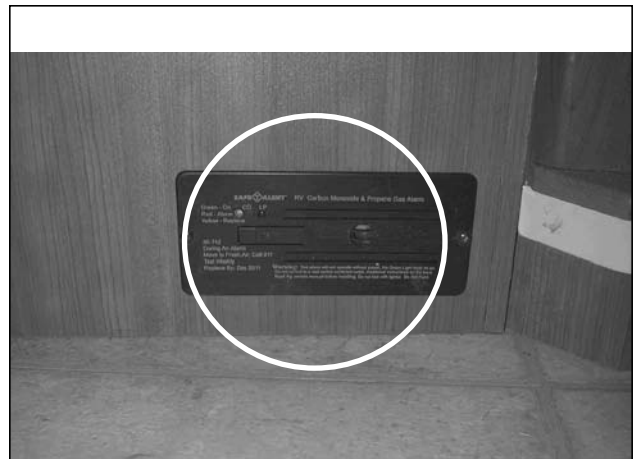
Picture F-P1: Propane/Carbon Monoxide detector.
