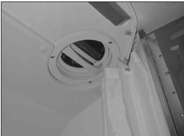
Picture B-P26: Bathroom exhaust vent.
