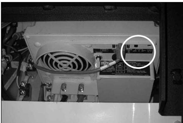
Picture B-P54: Location of inverter and Auto-Off-Charge Only switch.
