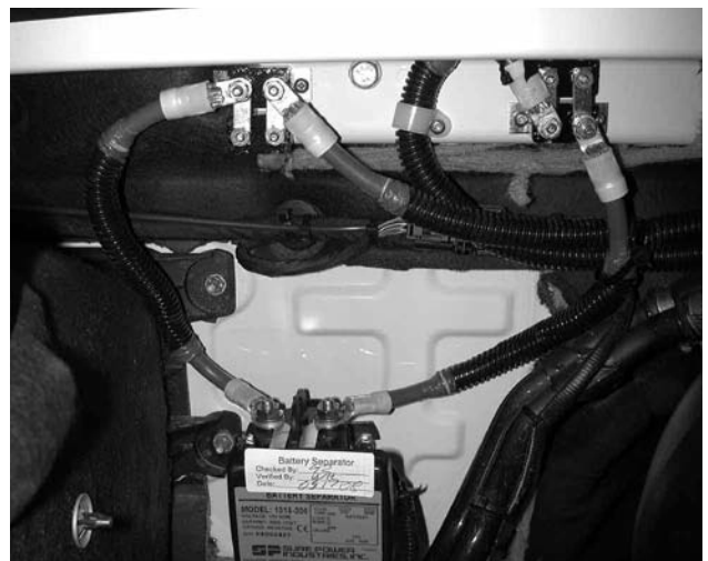
Picture B-P47: Battery Separator and breakers
