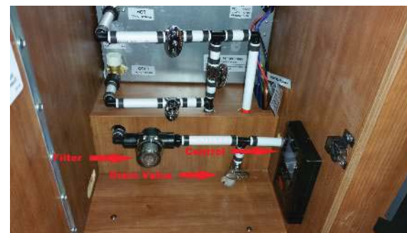
Tankless water heater drains
