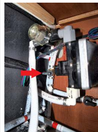
Third water heater bypass valve
