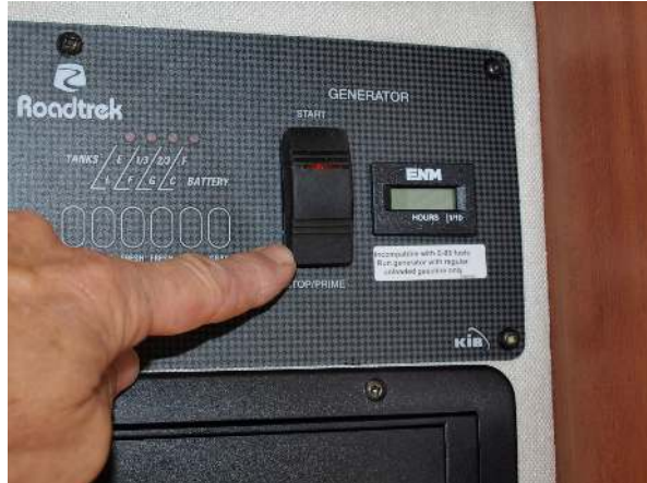
Generator switch, prime/off position
