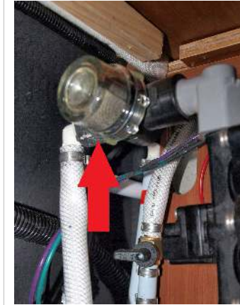
Water pump filter
