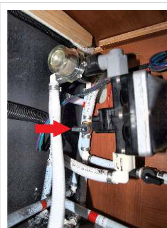
Third water heater bypass valve
