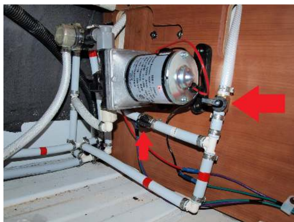
First two water heater bypass valves
