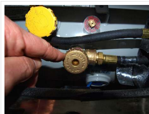
Propane tank main shutoff valve
