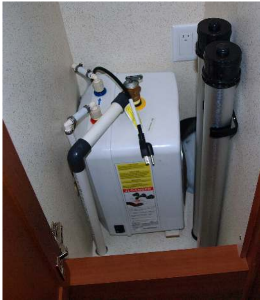
Electric water heater
