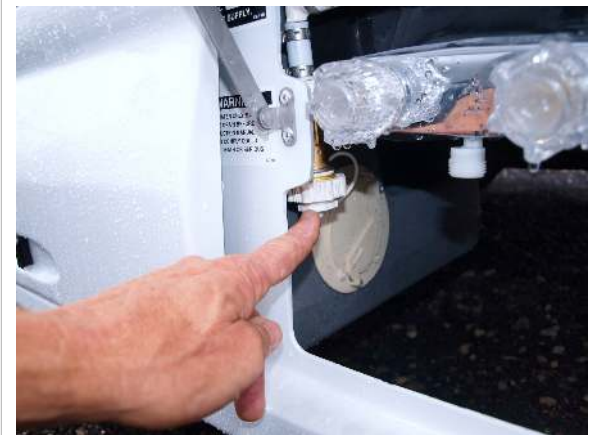
City water connection
