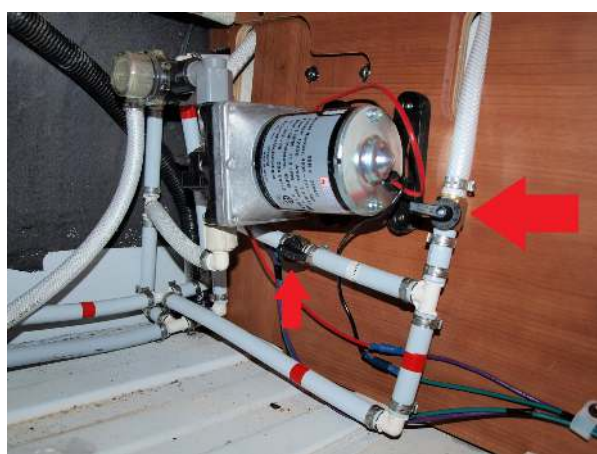
First two water heater bypass valves
