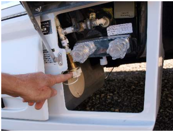
City water fill location
