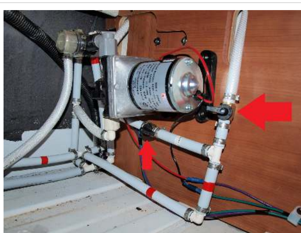
Water heater bypass valves
