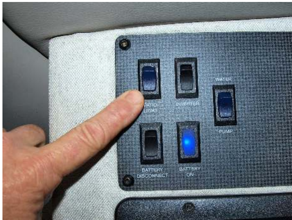
Patio light switch
