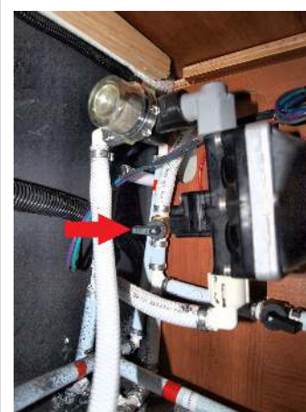
Third water heater bypass valve
