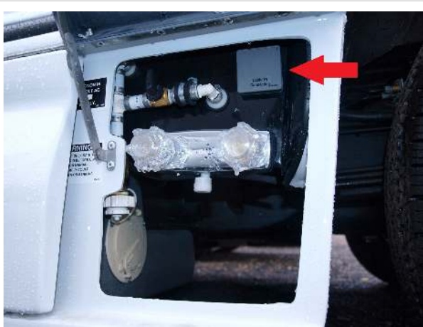
Cable TV connection location
