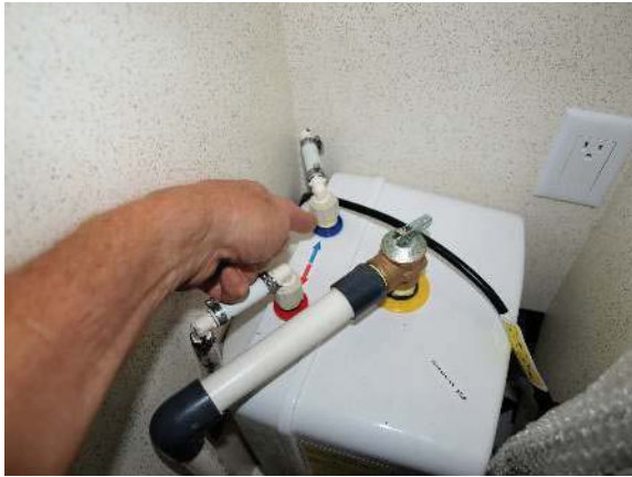
Water heater fittings
