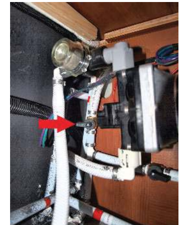
Third water heater bypass valve
