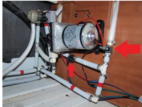
First two water heater bypass valves
