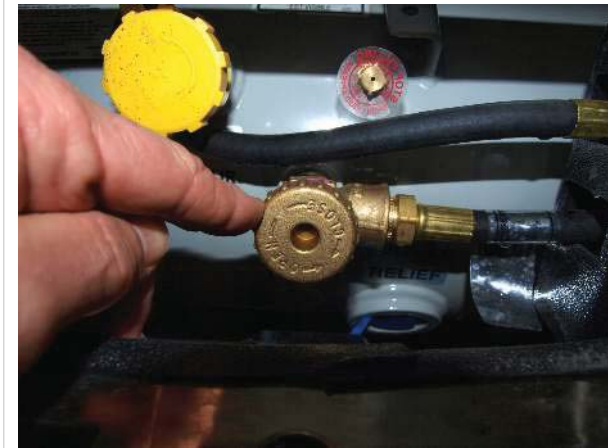
Propane tank main shutoff valve
