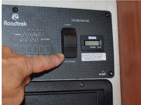
Generator switch, prime/off position
