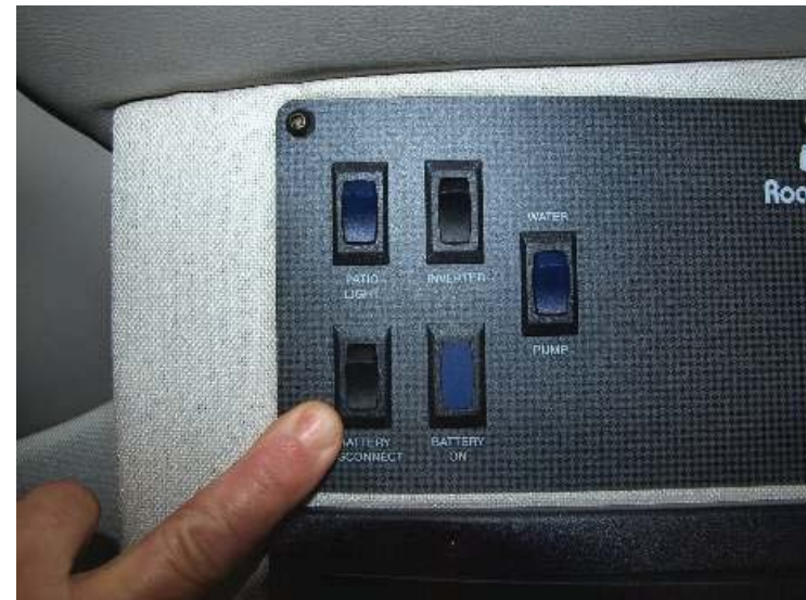
Battery disconnect switch
