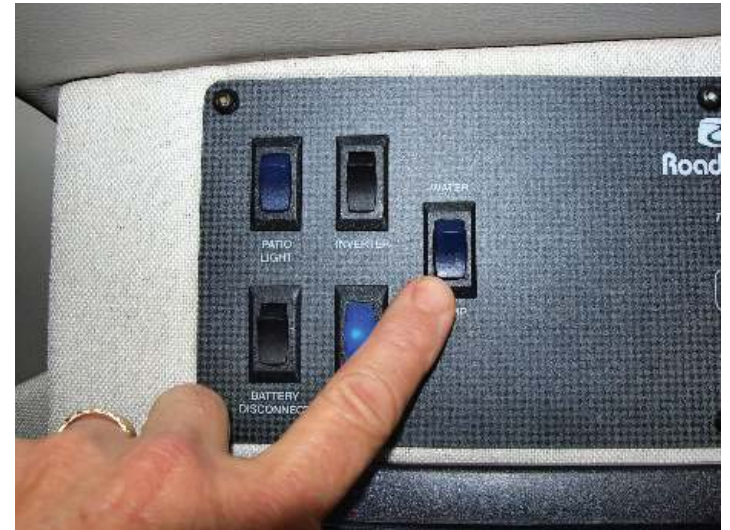
Water pump switch
