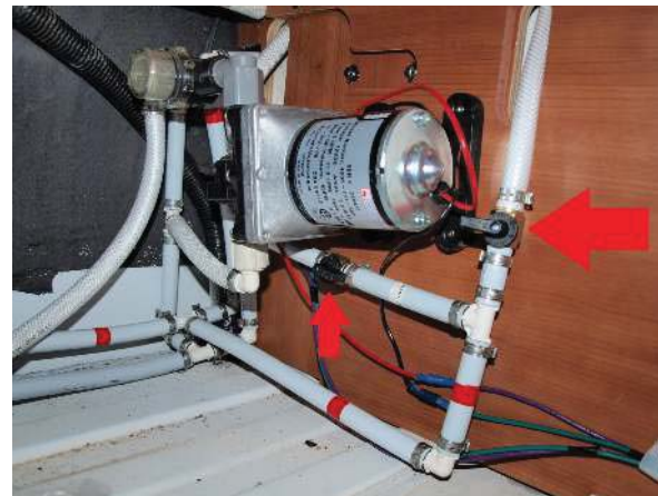
Water heater bypass valves
