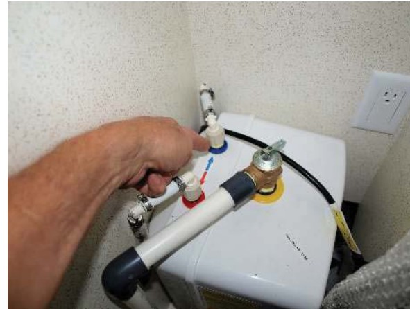
Water heater fittings
