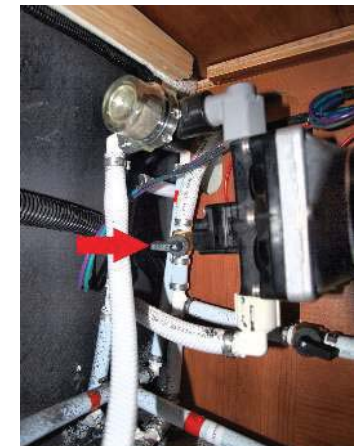
Third water heater bypass valve
