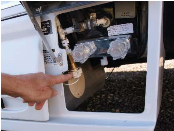
City water fill location
