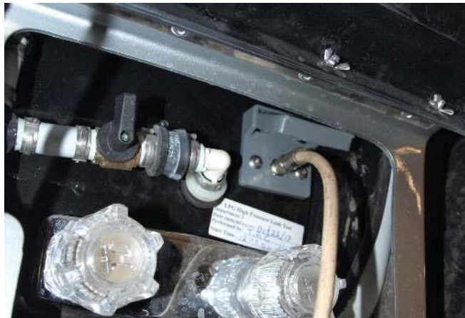
TV cable connected
