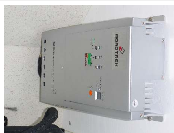
Solar controller in cabinet above galley
