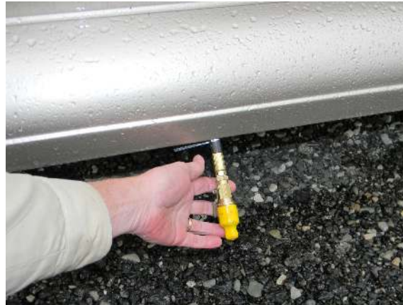
Propane pigtail, removed from retaining enclosure
