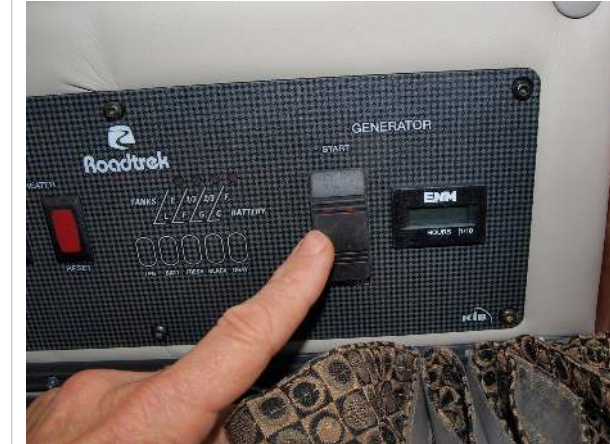
Propane generator switch and hour meter
