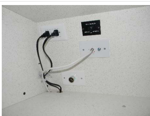
TV antenna and cable connections
