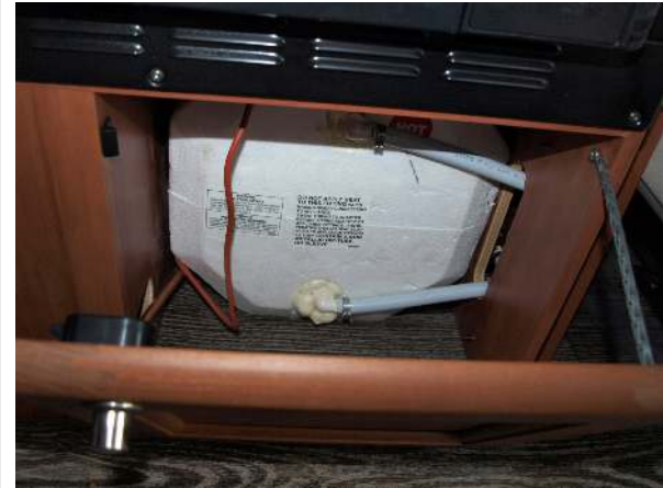
Water heater enclosure, under microwave convection oven
