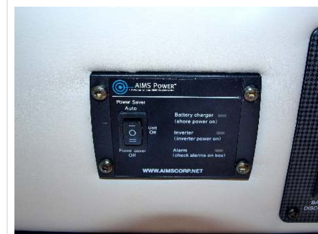
Inverter Control Panel
