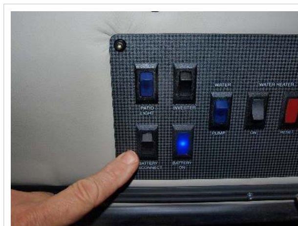
Battery disconnect switch
