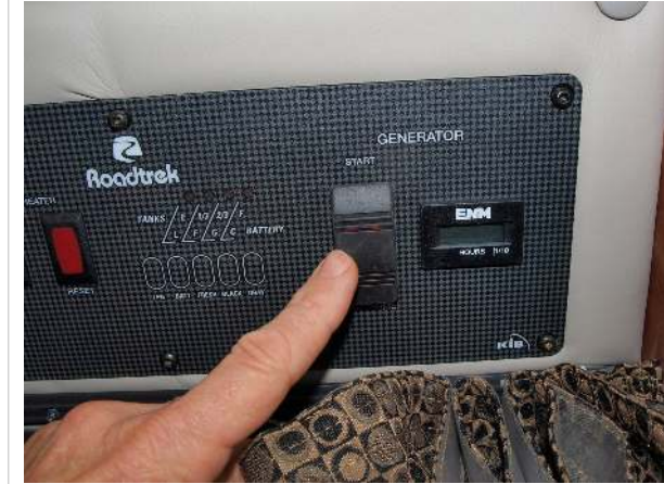
Propane generator switch and hour meter
