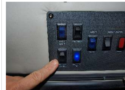
Battery disconnect switch
