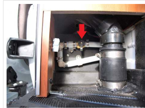
City water connection valve, shown closed
