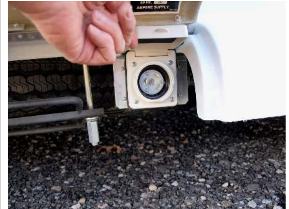
Shore power connection
