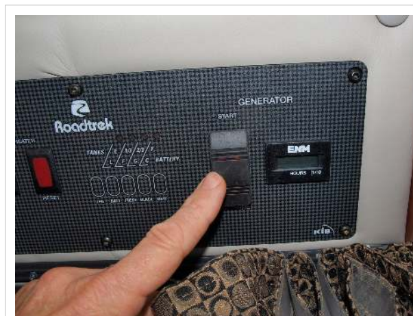
Propane generator switch and hour meter
