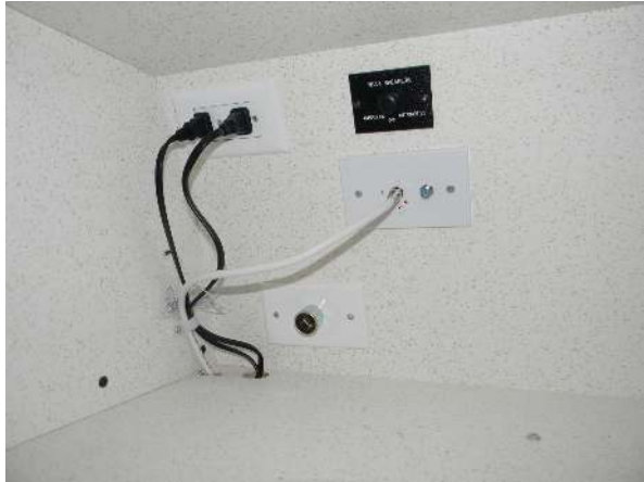
TV antenna switch and power injector
