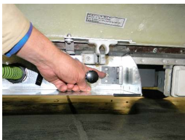
Cable TV connection location
