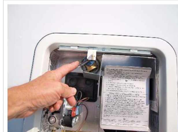
Water heater pressure relief valve
