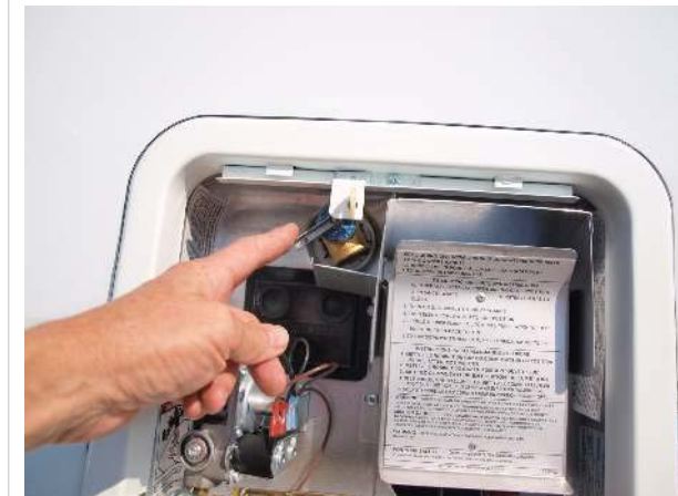
Water heater pressure relief valve
