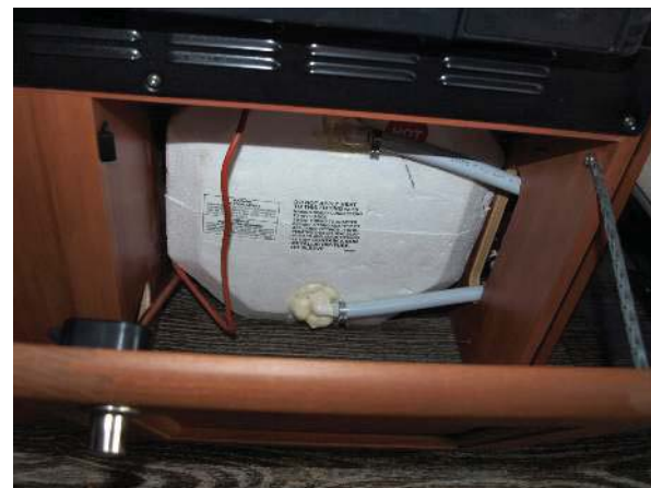
Water heater enclosure, under microwave convection oven
