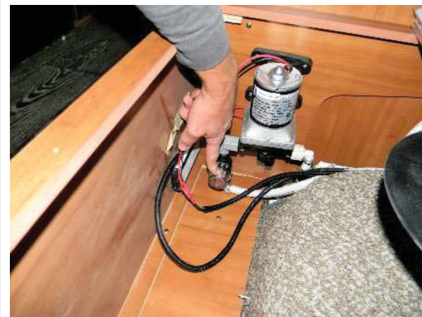
Water pump filter
