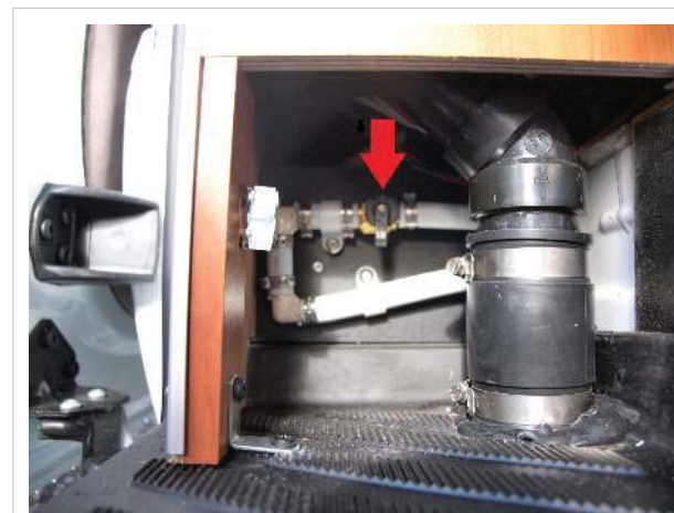
City water connection valve, shown closed
