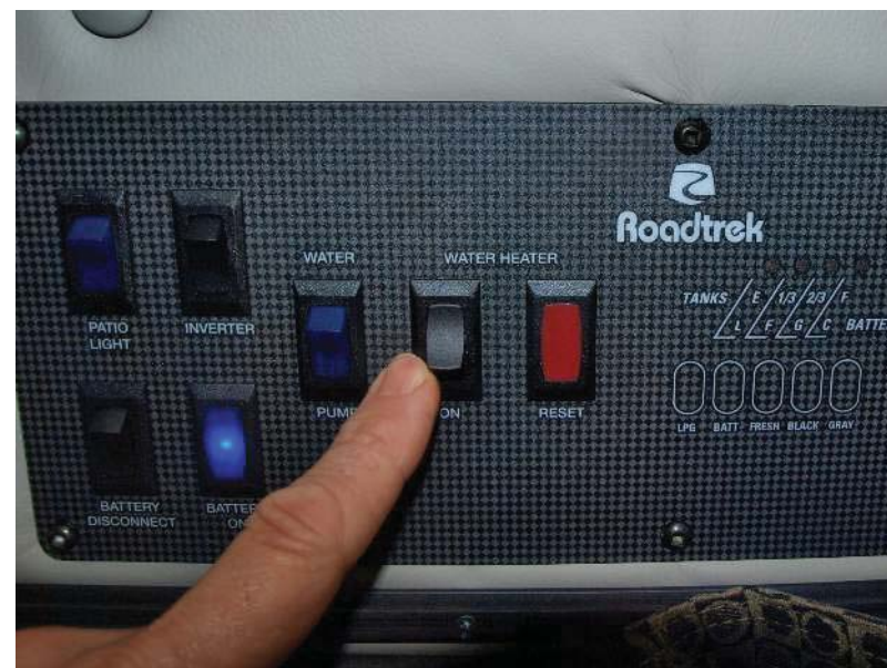
Water heater switch
