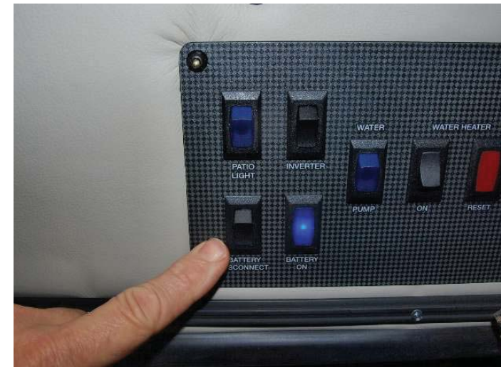
Battery disconnect switch on
