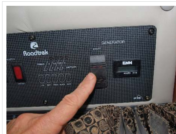
Propane generator switch and hour meter
