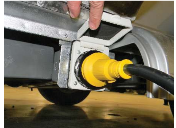
Attached shore power cord
