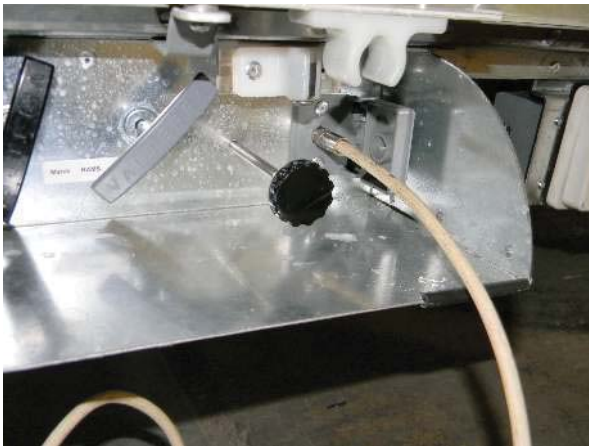
TV cable connected
