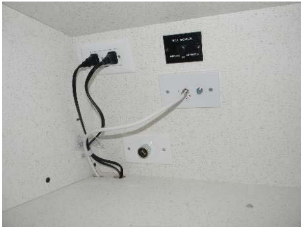
TV antenna switch and power injector
