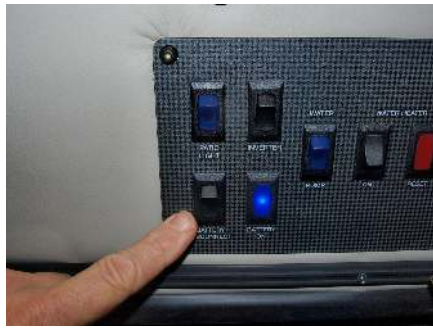
Battery disconnect switch
