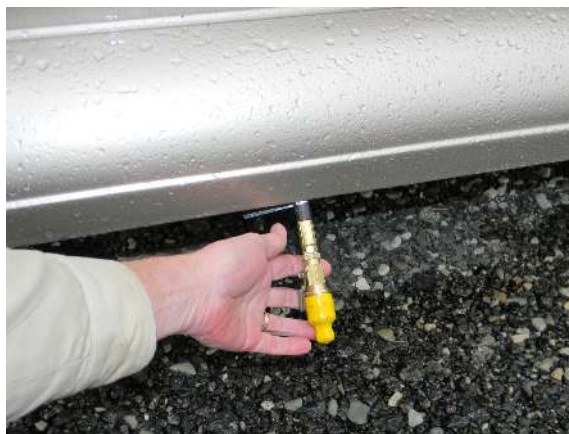
Propane pigtail, removed from retaining enclosure
