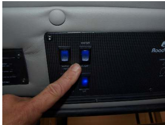
Water pump switch
