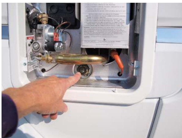
Anode rod location
