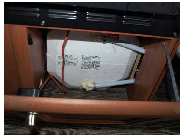
Water heater enclosure, under microwave convection oven
