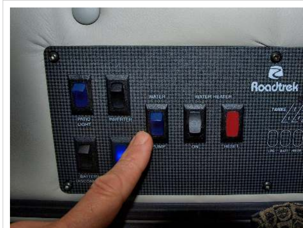
Water pump switch
