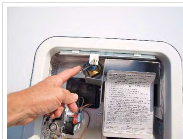
Water heater pressure relief valve
