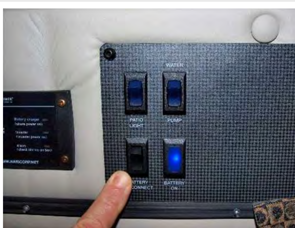
Battery disconnect switch
