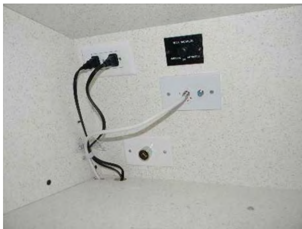
TV antenna and cable connections
