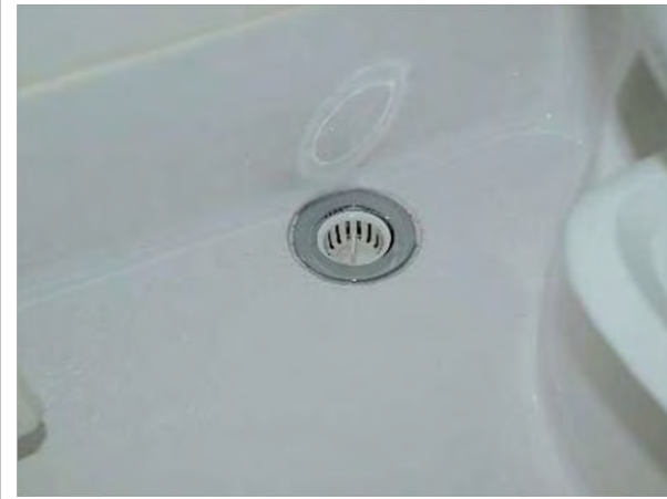
Shower floor drain plug
