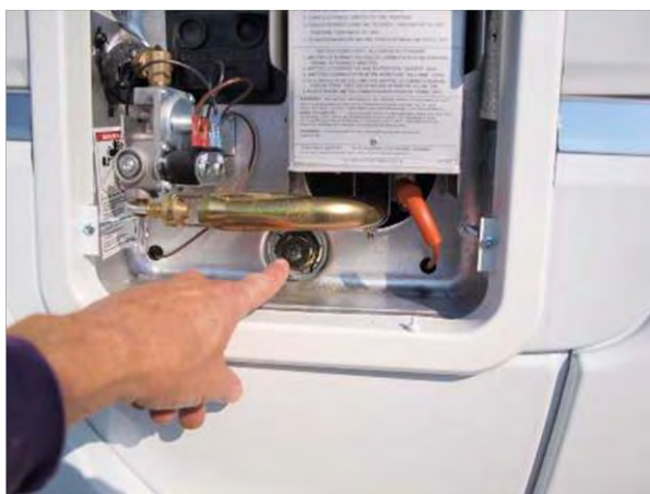
Anode rod location
