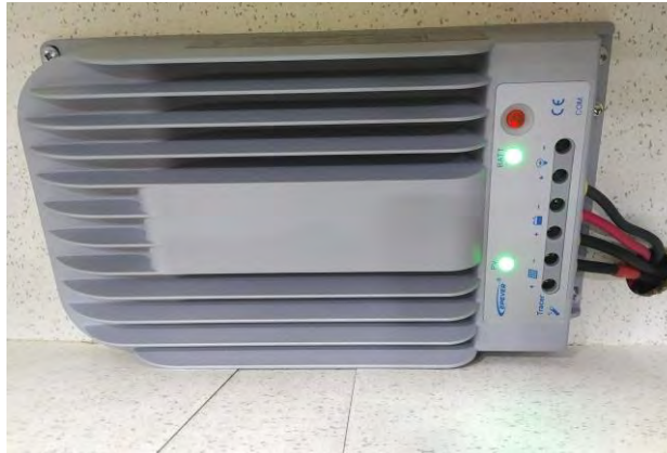
Solar controller in cabinet above galley
