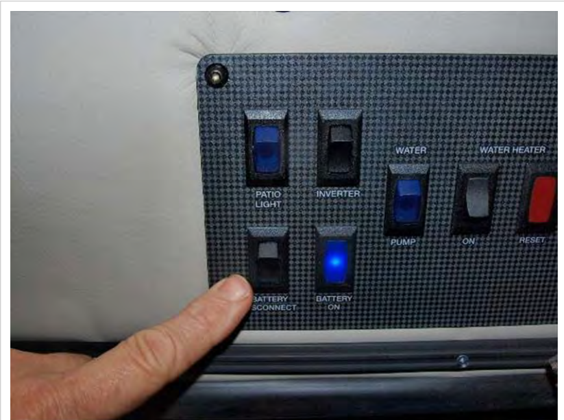
Battery disconnect switch on
