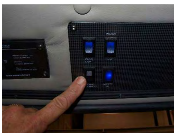
Battery disconnect switch
