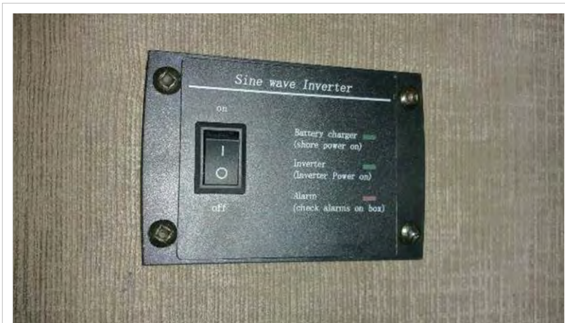
Inverter Control Panel
