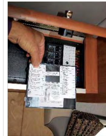
Agile AC breakers and 12-volt fuses
