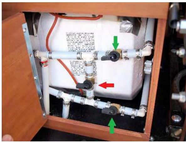
Water heater bypass valves in the normal position, all pointing to the left. Green means open, red closed.
