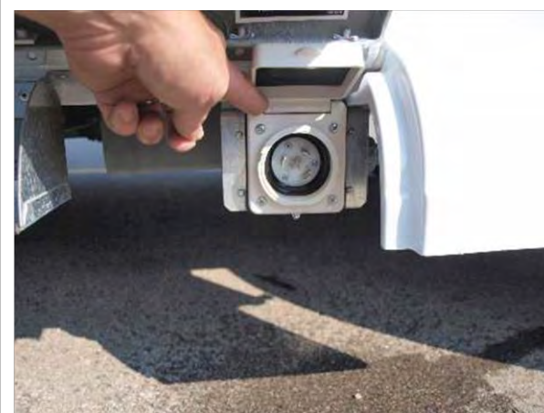
Shore power connection
