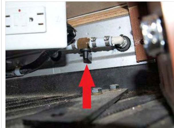
City water valve in shut position
