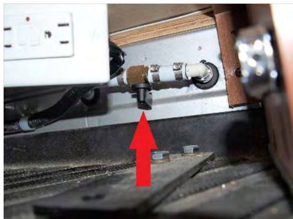
City water connection valve, shown closed
