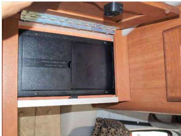
Agile power distribution panel location
