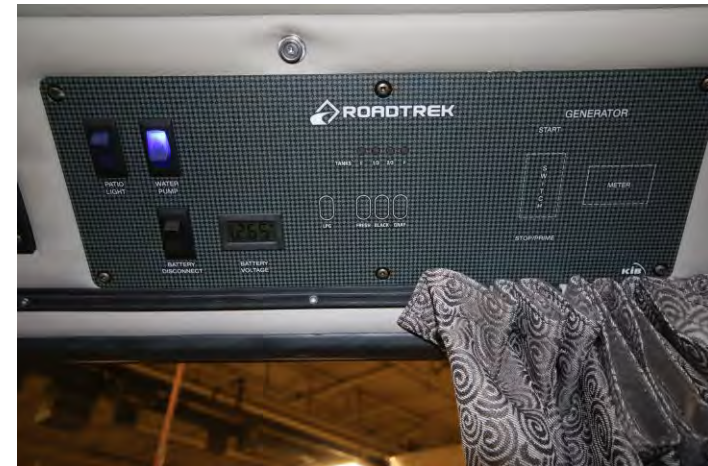
Monitor panel for units propane generator
