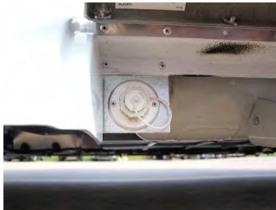
City water connection
