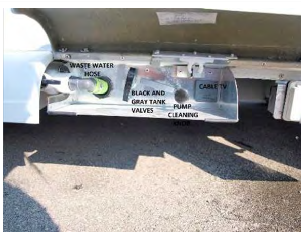
Wastewater hose, dump valves, pump cleaning knob, and CATV connection
