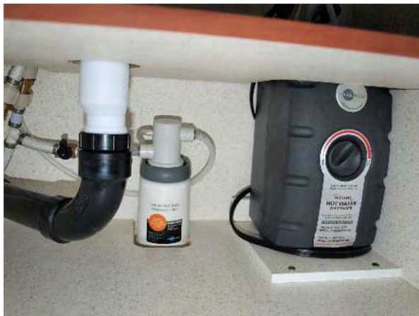
On-demand hot water system filter
