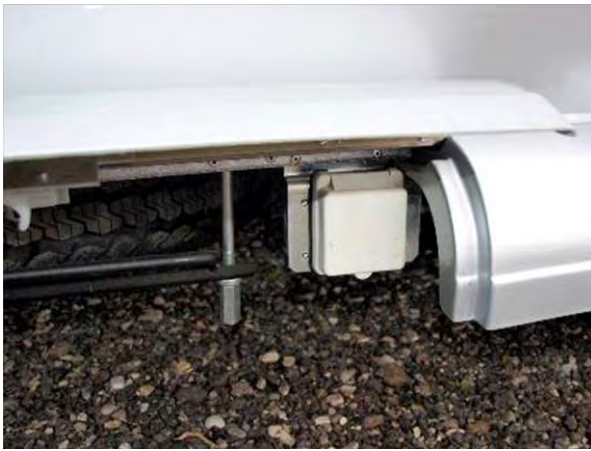
Shore power connection point
