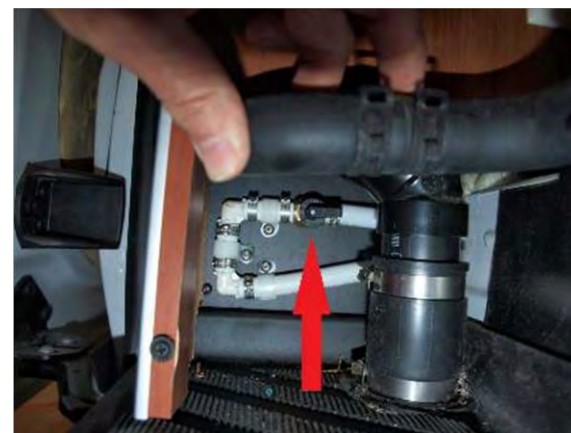
City water valve in open, along-the-line position
