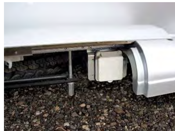
Shore power connection
