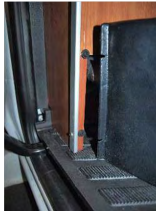
Screws holding plastic radiator cover on
