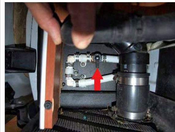
City water valve in closed, across-the-line position
