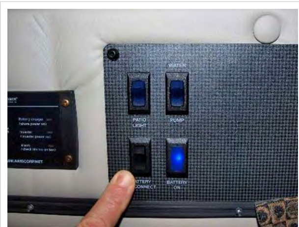
Battery disconnect switch
