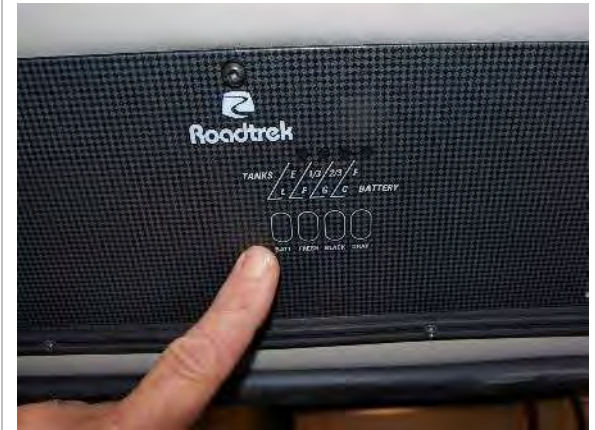
Tank and battery level indicators
