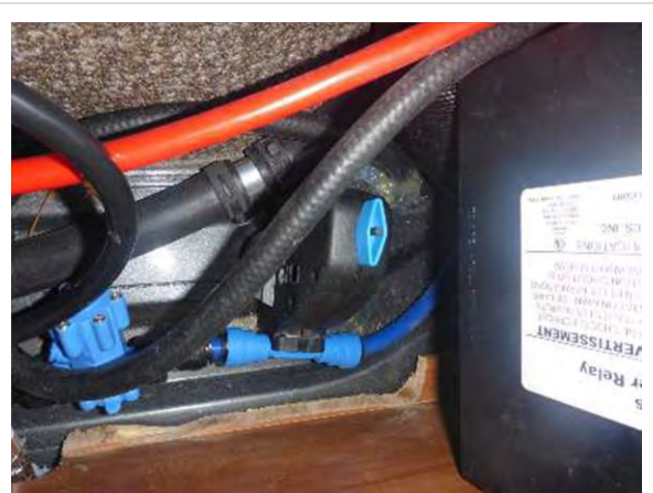
Frost control valve in tripped position
