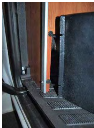
Screws holding plastic radiator cover on
