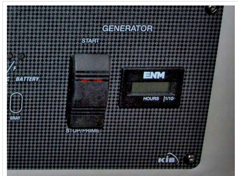
Propane generator control
