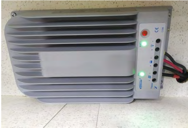
Solar controller in cabinet above galley
