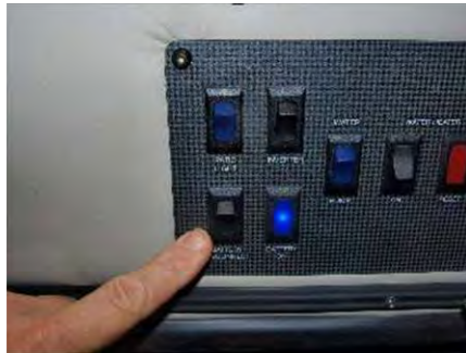
Battery disconnect switch
