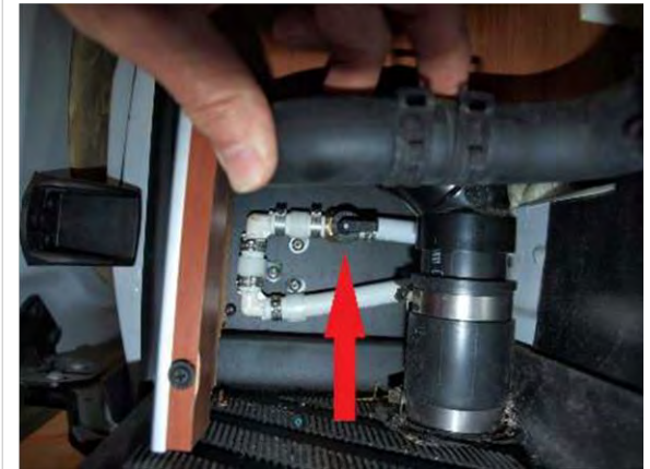
City water valve in open, along-the-line position
