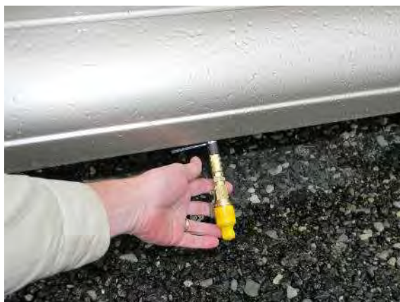
Propane pigtail, removed from retaining enclosure
