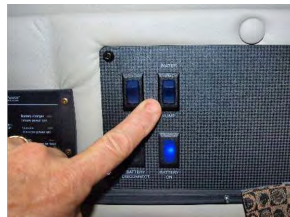
Water pump switch with 2500 watt inverter
