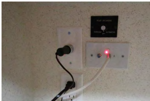
TV antenna and cable connections
