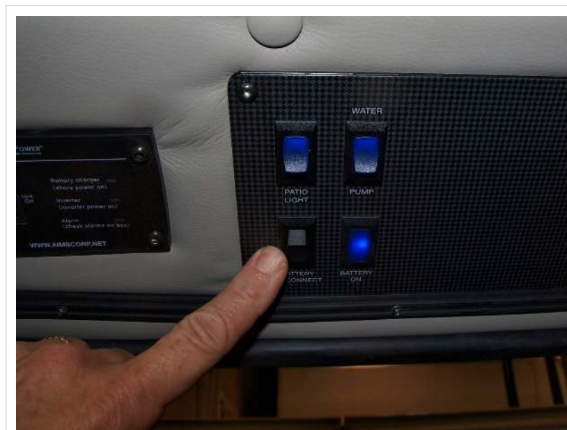
Battery disconnect switch
