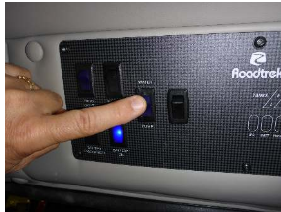
Water pump switch
