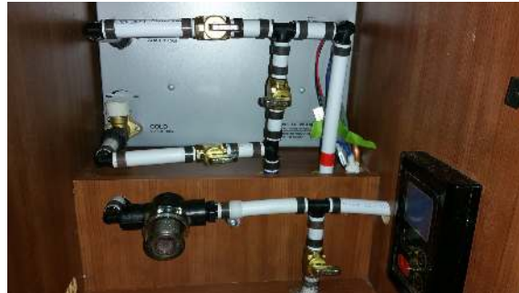
Water heater thermostat, filter and drain valves
