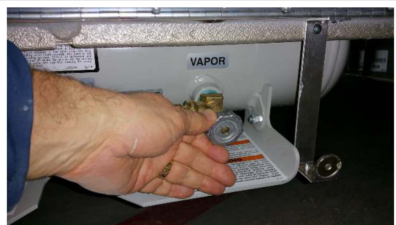
Propane tank main shutoff valve
