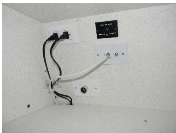
TV antenna switch
