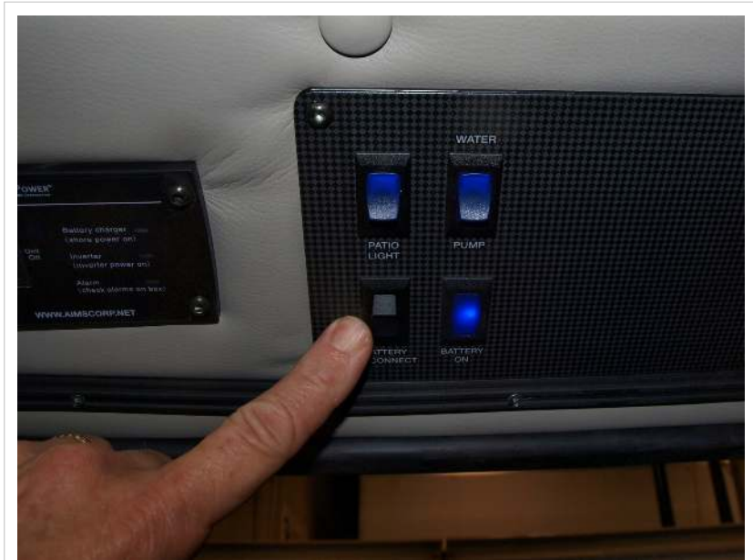
Battery disconnect switch
