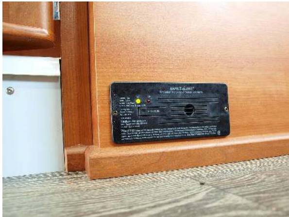
Propane and Carbon Monoxide alarm
