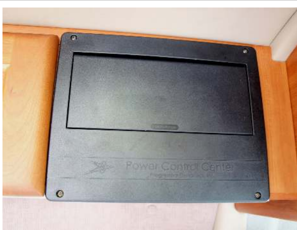
120VAC breaker panel
