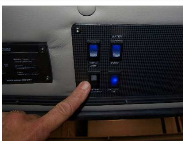
Battery disconnect switch
