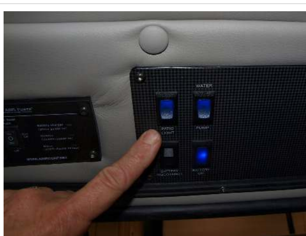
Patio light switch
