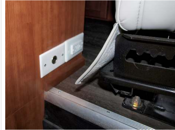
GFCI outlet behind rear captain's seat
