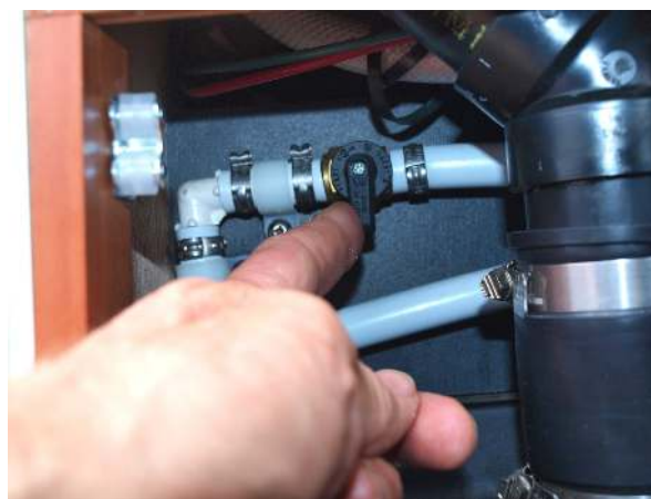
City water valve in closed, across-the-line position
