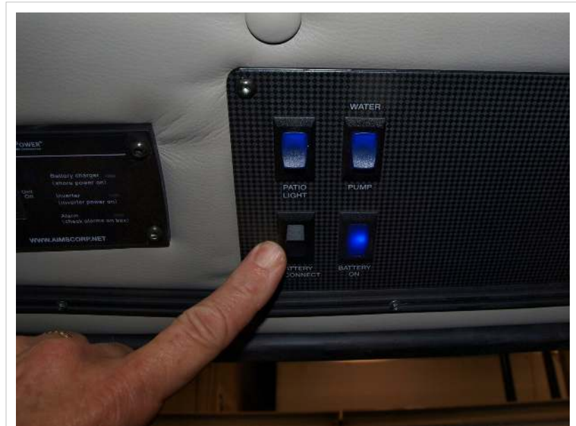
Battery disconnect switch
