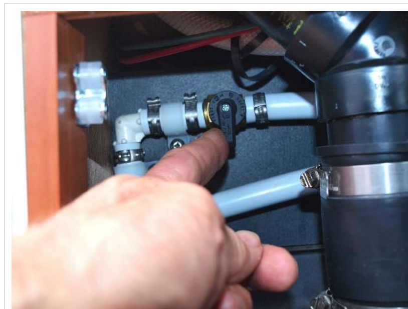
City water valve (shown closed)
