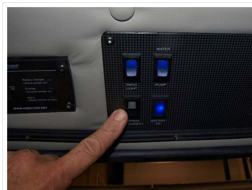
Battery disconnect switch
