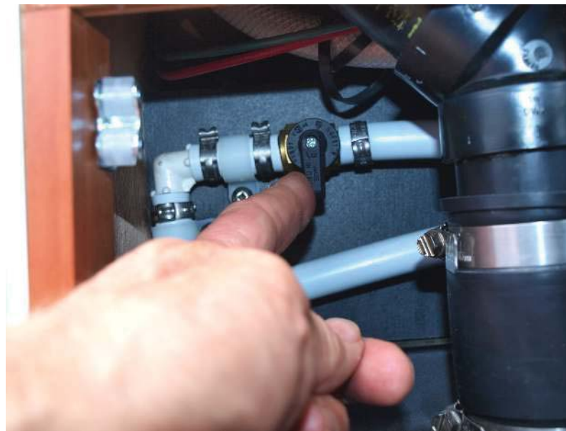
City water valve (shown closed)
