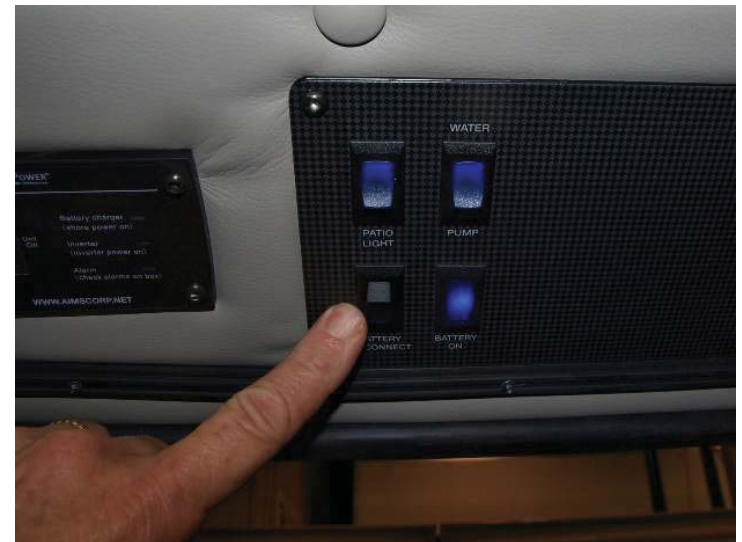
Battery disconnect switch
