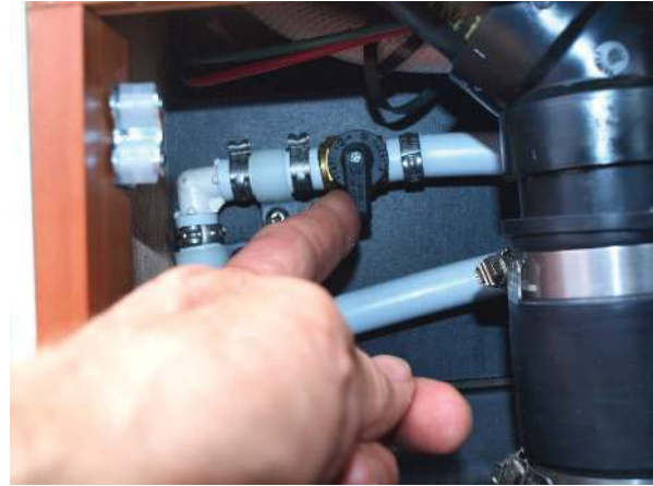
City water valve in closed, across-the-line position
